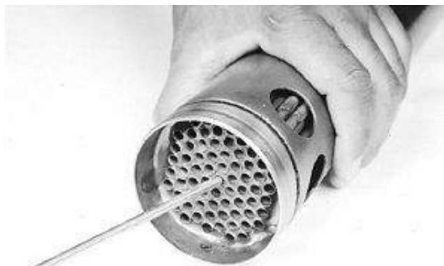
Clean Heat Exchanger
