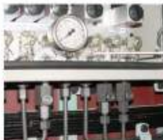
Fig. 3) Damper and pressure gauge
