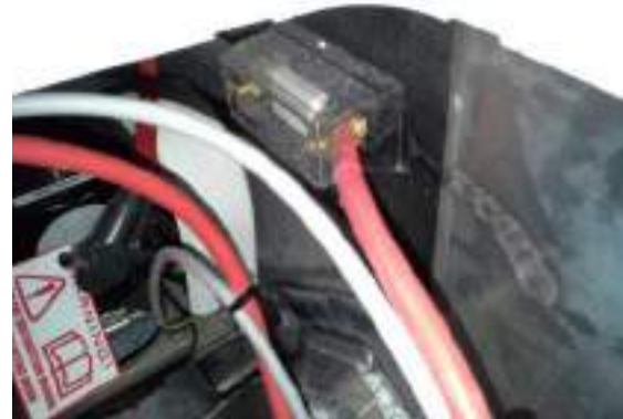
Figure 24. The bow thruster motor and its electrical connections.
