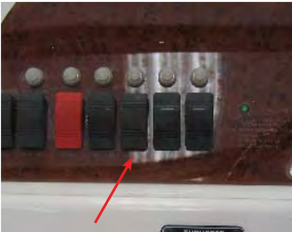
The Navigation/Anchor Light switch is located at the Helm Station.
