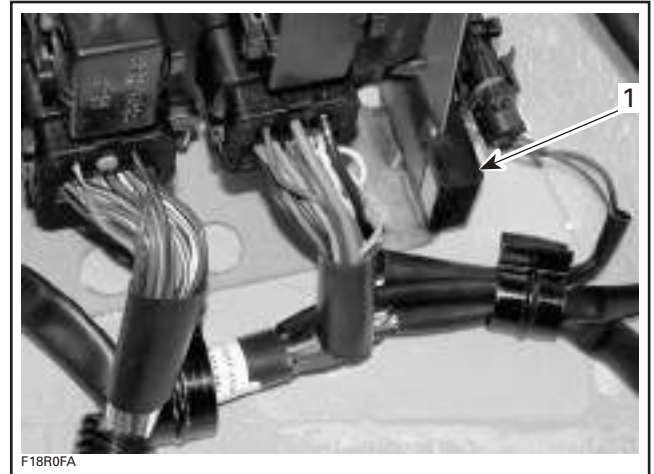
TYPICAL 1. Tops switch
