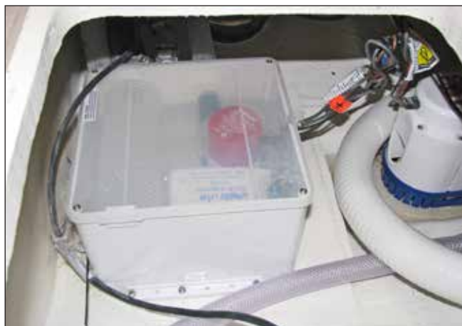
Sump Pump System In Forward Bilge
