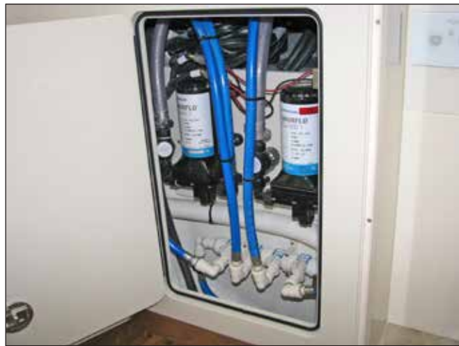
Fresh Water Pump Access Panel In Shower
