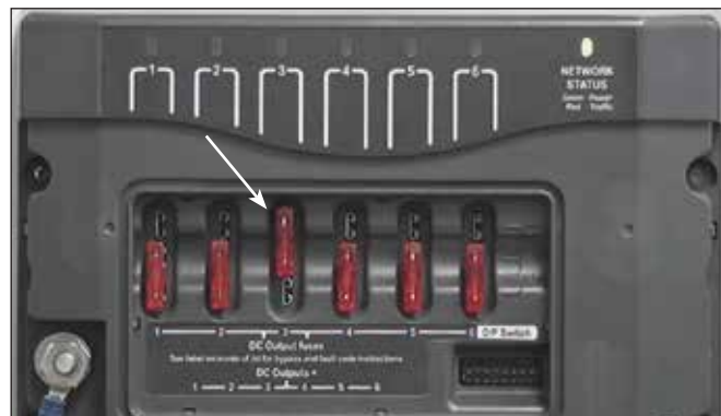
CZone Circuit 3 Fuse In Bypass Position
