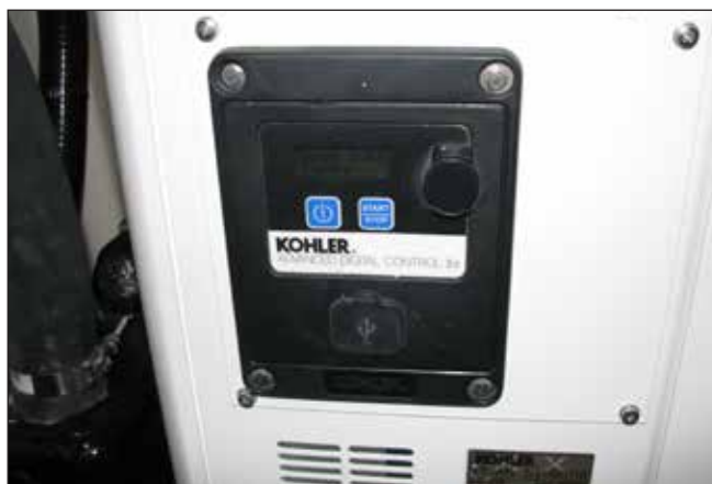
Generator Onboard Control Panel
