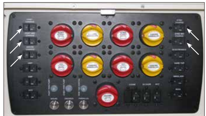
Battery/Charger Circuit Breakers
