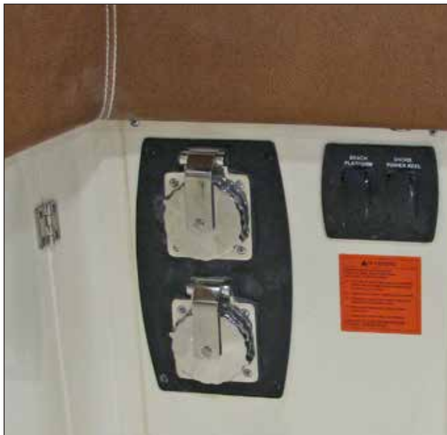
Shore Power Inlet Breaker & ELCI Inlet Panels
