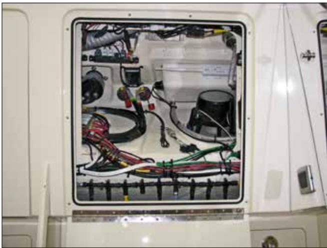
Helm Access Panel Above Marine Toilet
