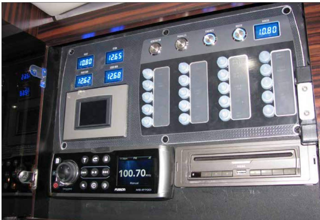
Cabin DC Breaker Panel, Stereo, DVD Player & Air Conditioner Control Panel
