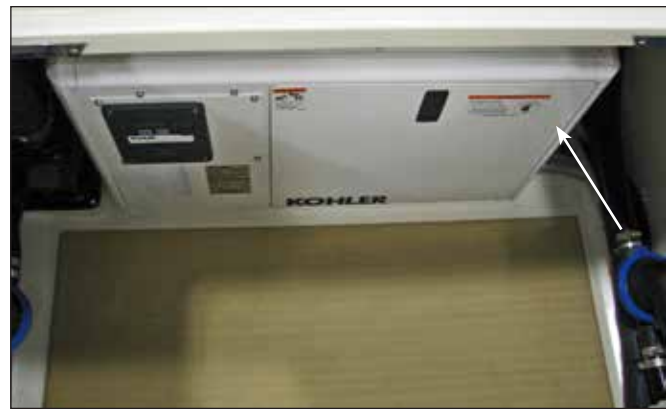
Diesel Generator Fuel Filter Location Behind Sound Shield Access Panel
