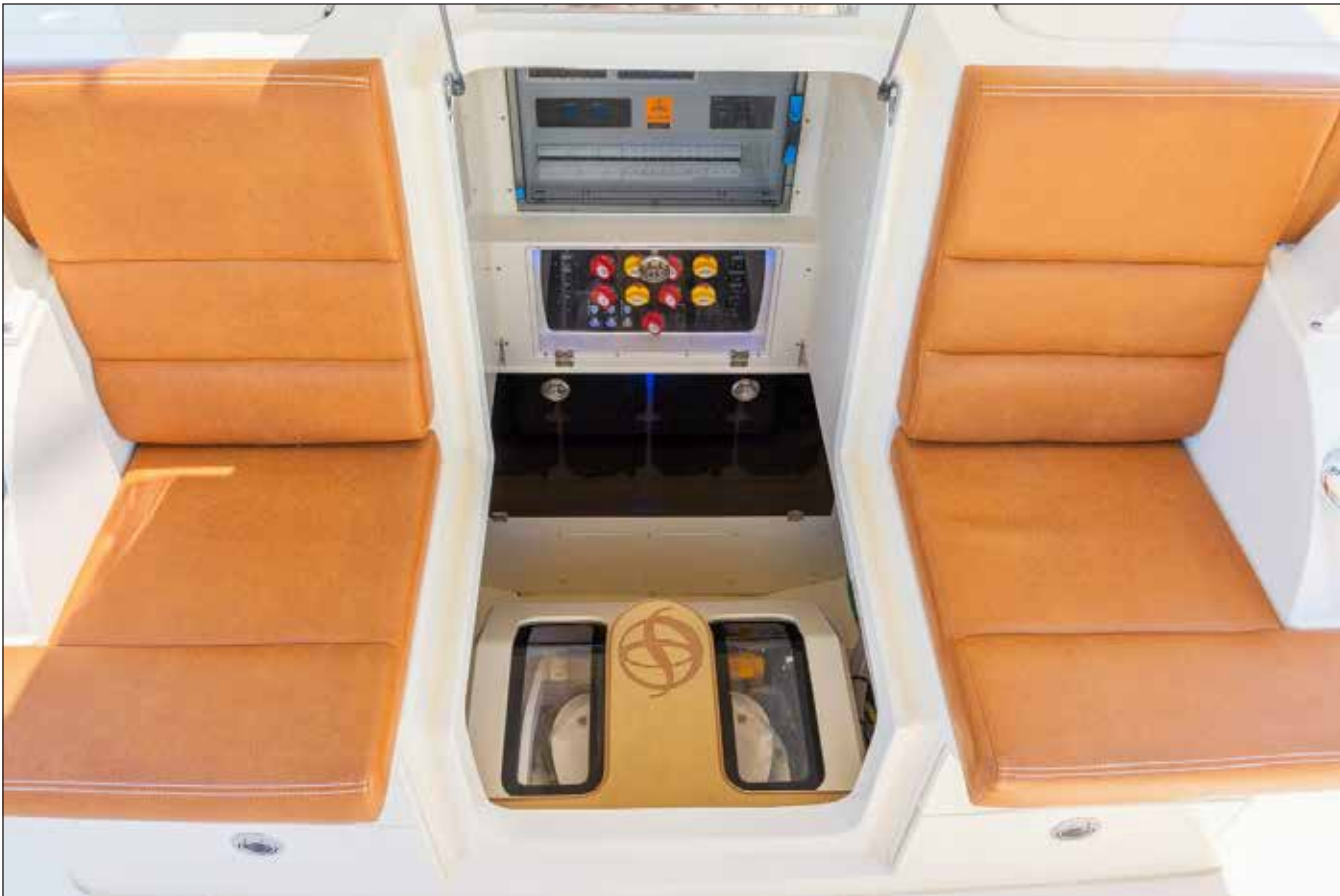
Electrical Systems Room & Battery Switch Panel Below Leaning Post/Helm Seats
