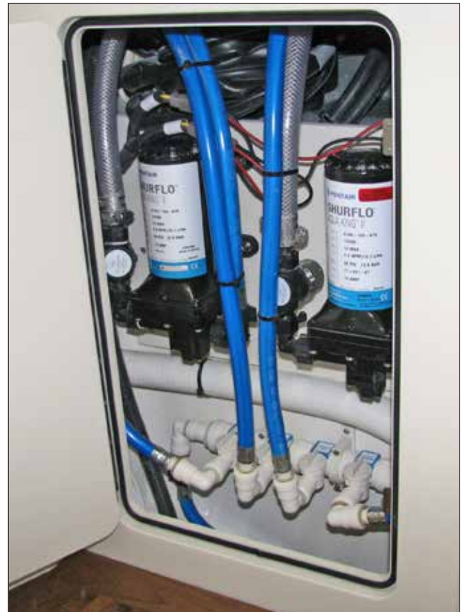
Fresh Water Pumps in the Aft Head Compartment Bulkhead
