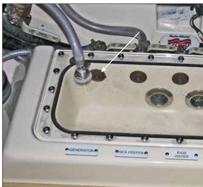
Generator Cooling Pump Supply Valve Fitting
