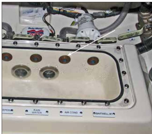
Air Conditioner Cooling Pump Supply Valve Fitting
