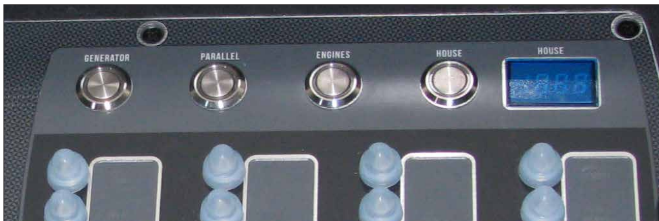
Cabin DC Panel Remote Battery Switches
