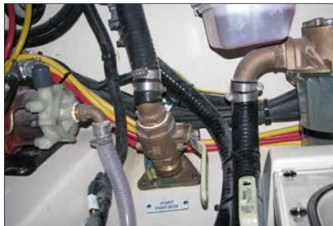
Port Fishbox Pump Out Thru-Hull Fitting & Valve
