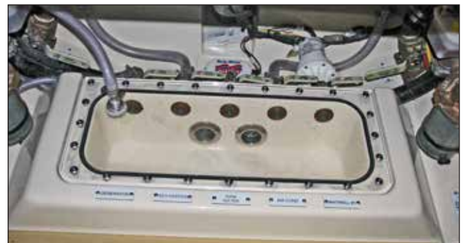
Generator Seawater Supply In Sea Chest
