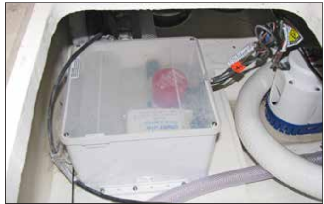
Shower Sump System In Head Compartment Bilge
