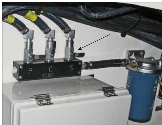
Stbd Engine Fuel Manifold & Valves
