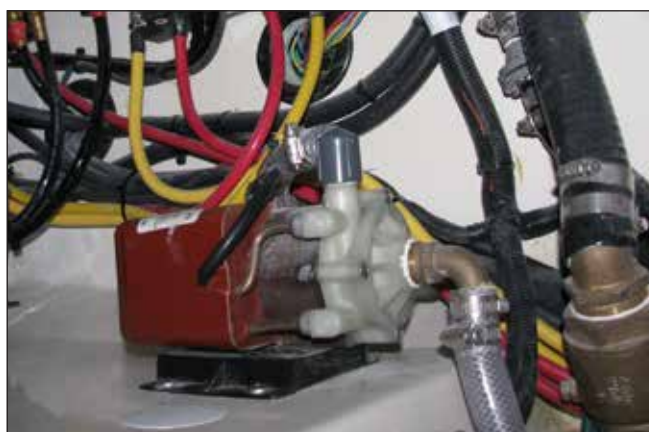
Air Conditioner Seawater Cooling Pump
