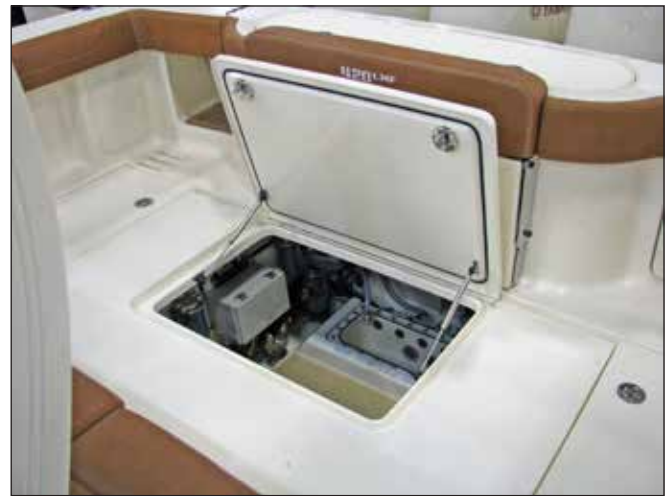
Aft Systems Room Hatch
