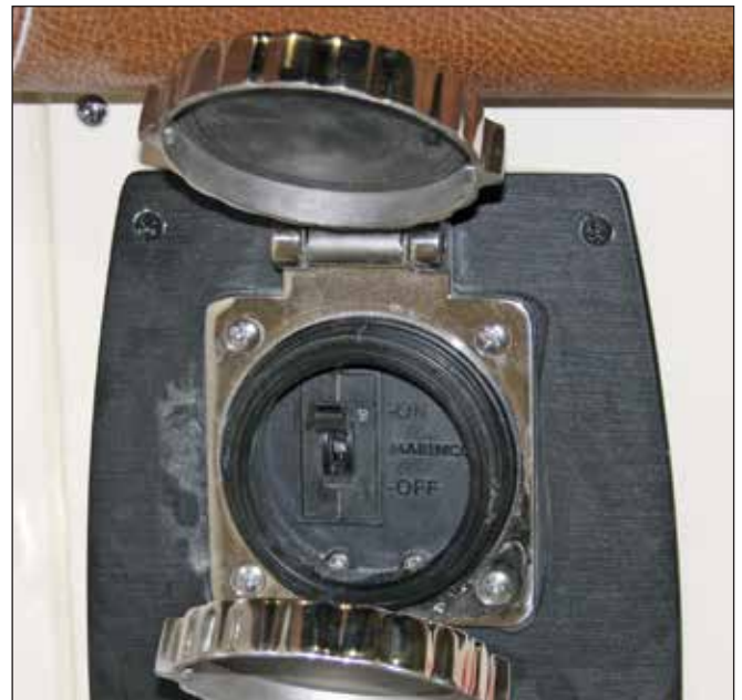
Shore Power Inlet Circuit Breaker
