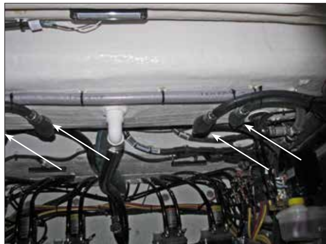
Fuel Primer Bulbs In Aft Systems Room
