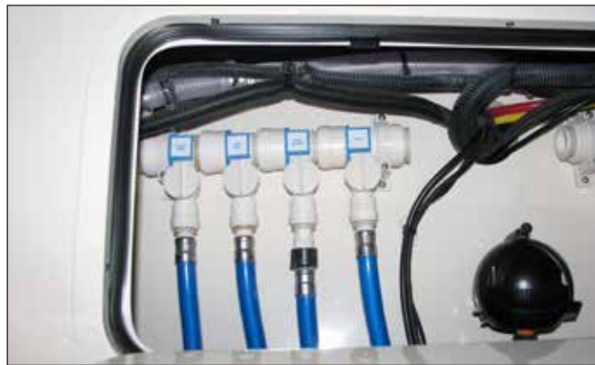
Cold Water Shutoff Valves Near Water Tank
