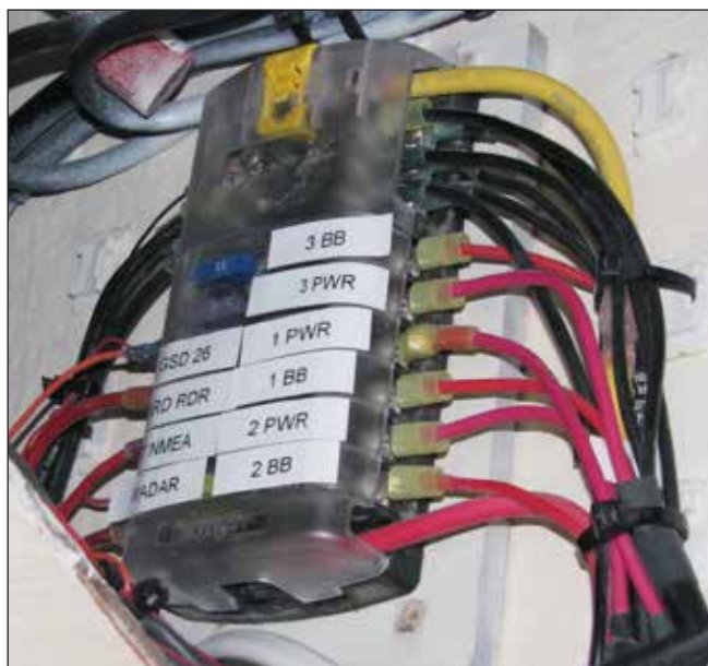
Electronics Fuse Panel
