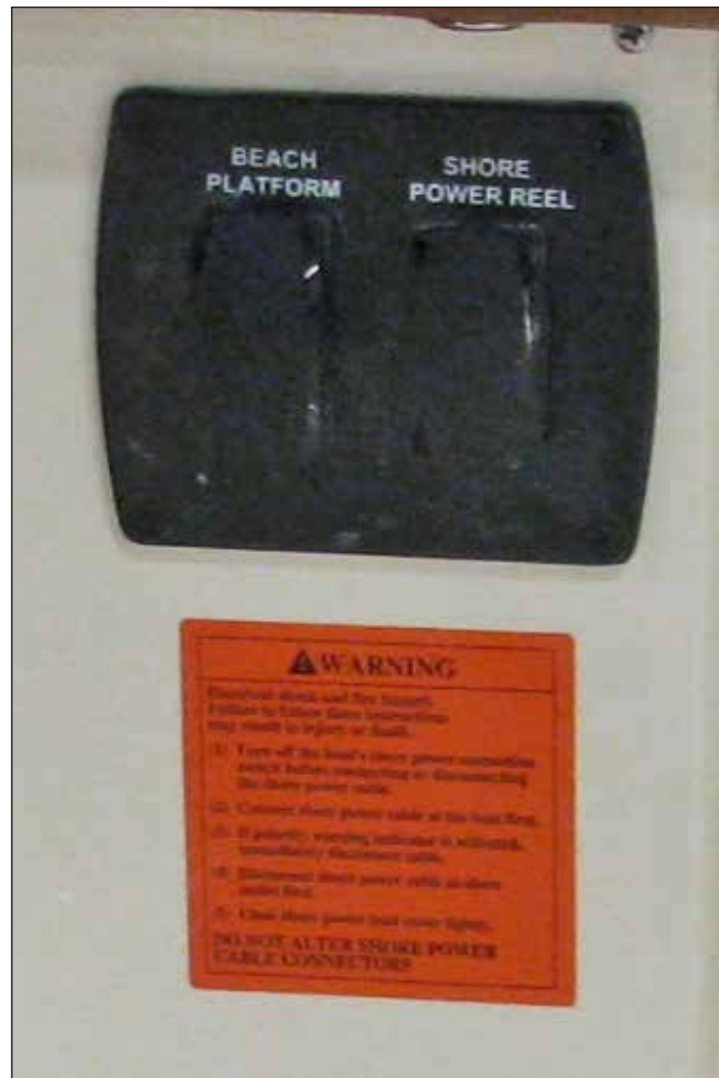
Shore Power Reel Switch
