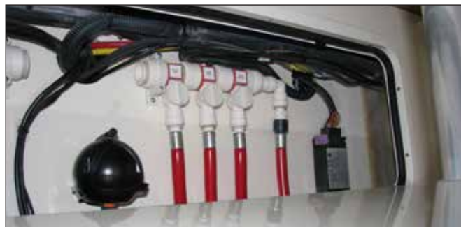
Hot Water Shutoff Valves Near Water Tank
