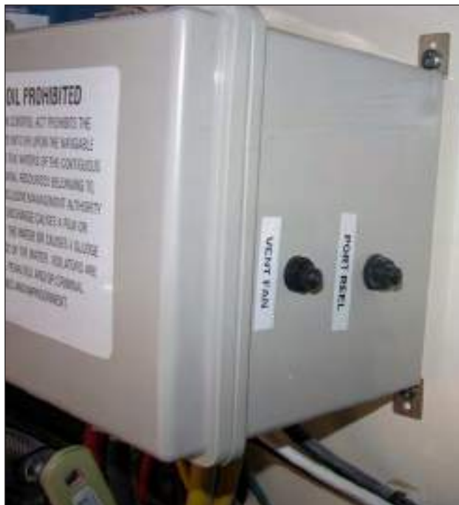
Port Side Electrical Box - Vent Fan & Port Electric Reel Circuit Breakers
