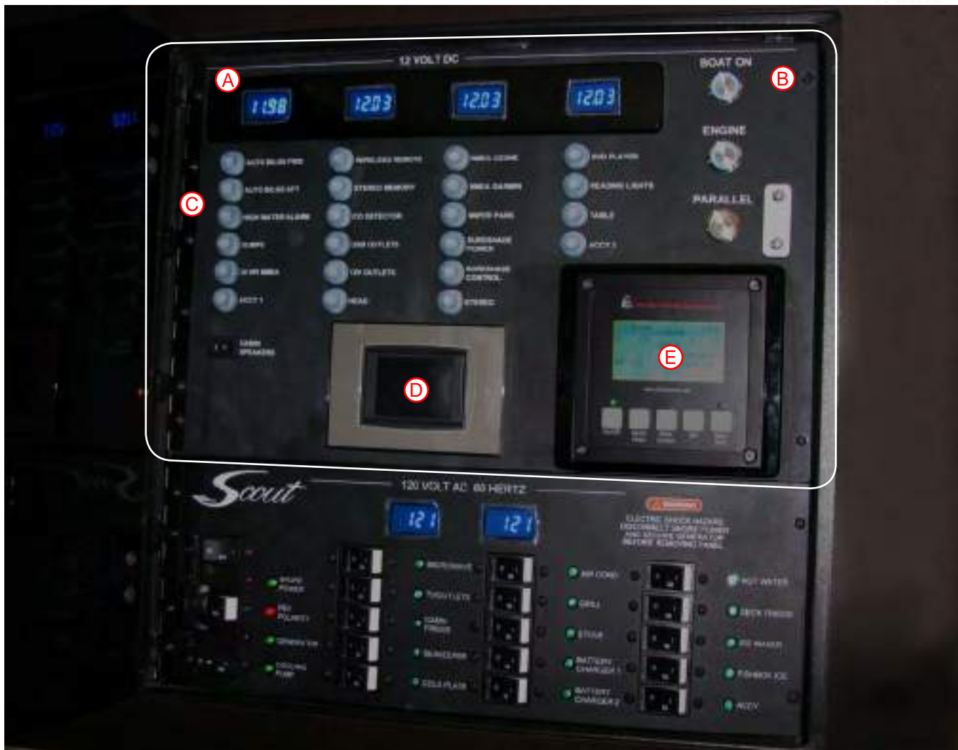
Cabin DC Breaker Panel, CZone Display & Generator Control Panel
