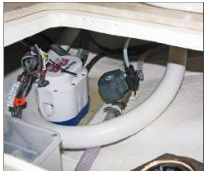
Forward Bilge Pump With Automatic Switch
