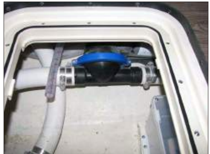
Diaphragm Discharge Pump & Waste Discharge Valve In Forward Cabin Bilge Below Dinette Table
