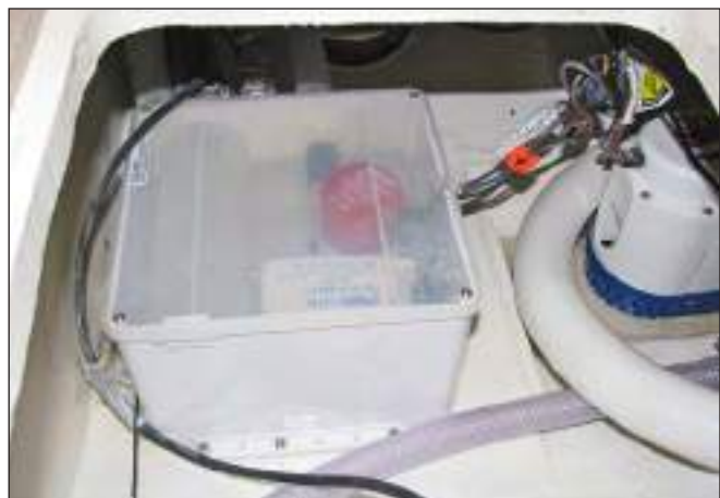
Typical Shower & Drain Sump Pump System In The Bilge Below The Head Compartment
