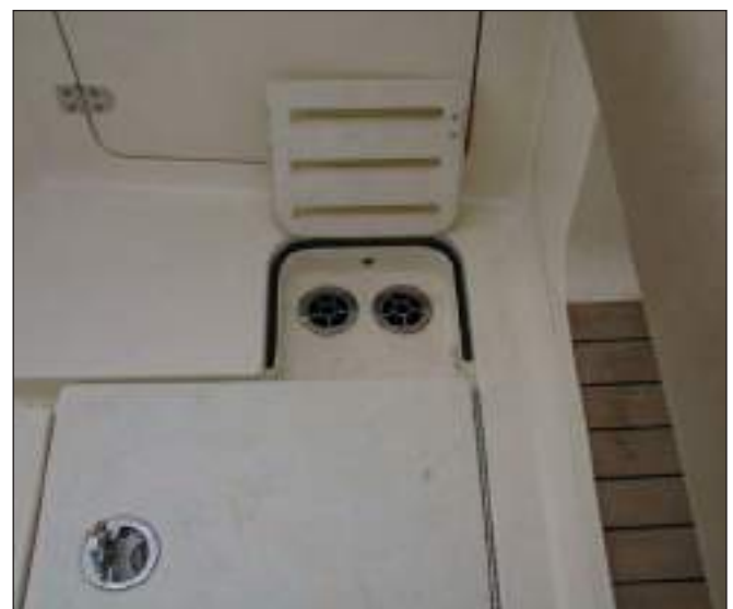
Scupper Drain Thru-Hull Fittings & Check Valves
