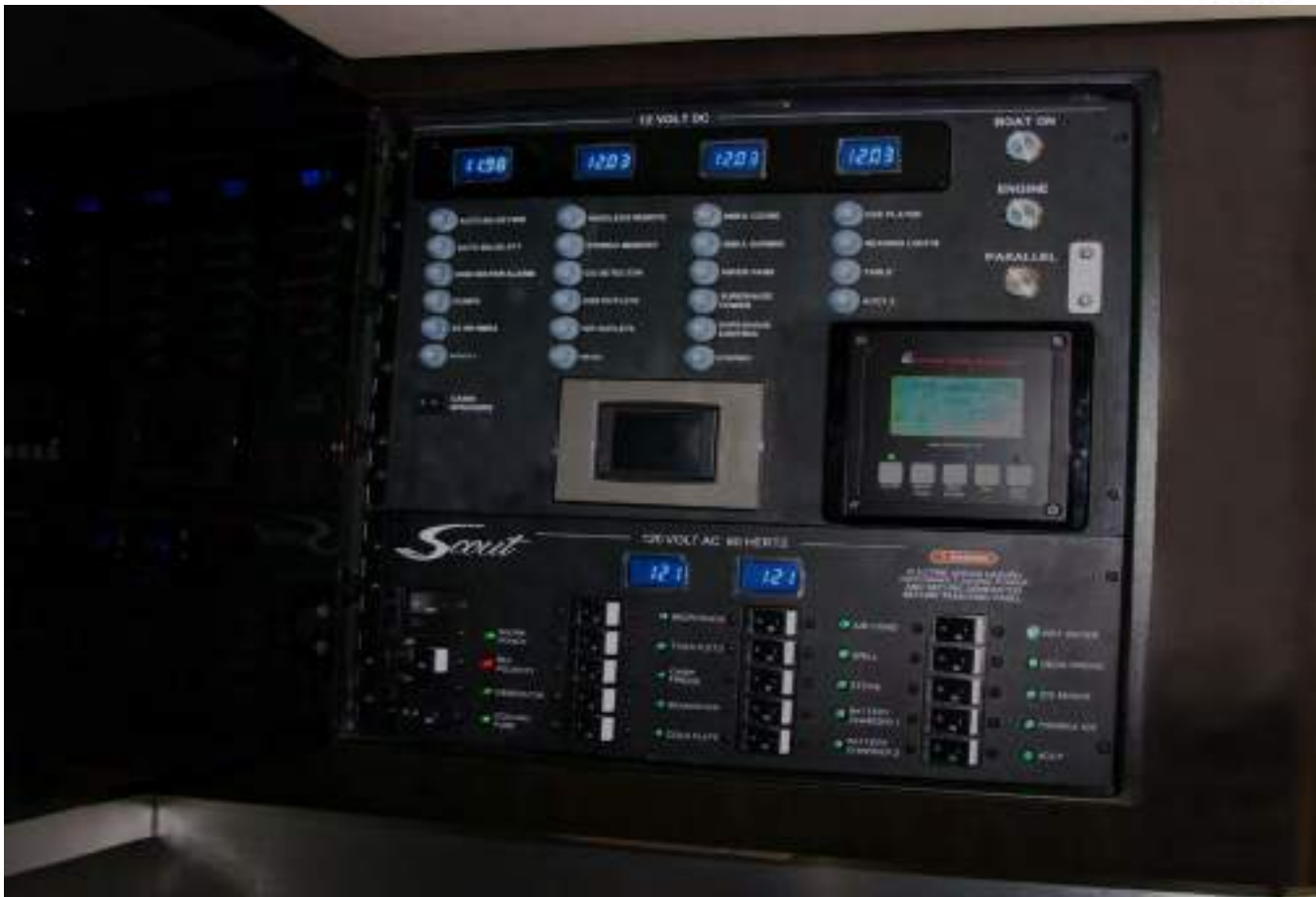
Cabin AC/DC Panel, Generator Control Panel & CZone Control Panel
