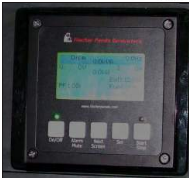
Typical Generator Control Panel
