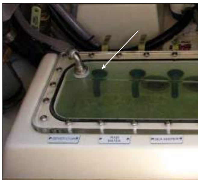
Generator Cooling Pump Supply Valve Fitting
