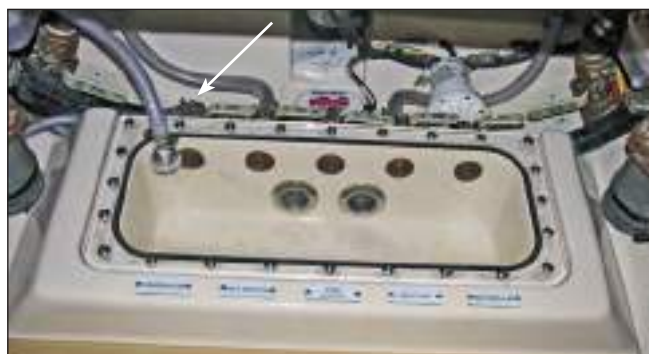
Generator Seawater Supply In Sea Chest
