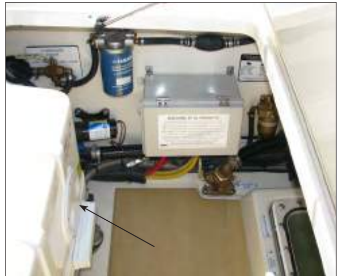
Diesel Generator Fuel Filter Location Behind Sound Shield Access Panel
