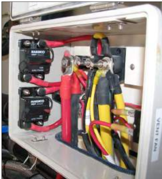
Electrical Box & Typical Yamaha Electronic Steering & Auxiliary Engine Charging Circuit Main Breakers
