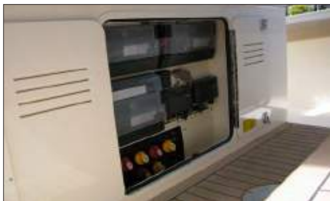
Battery Switch Panel, CZone Control Modules & Access Door
