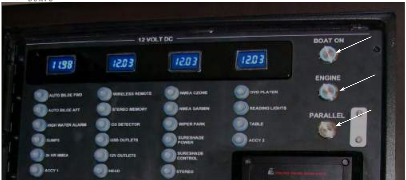
Cabin DC Panel Remote Battery Switches
