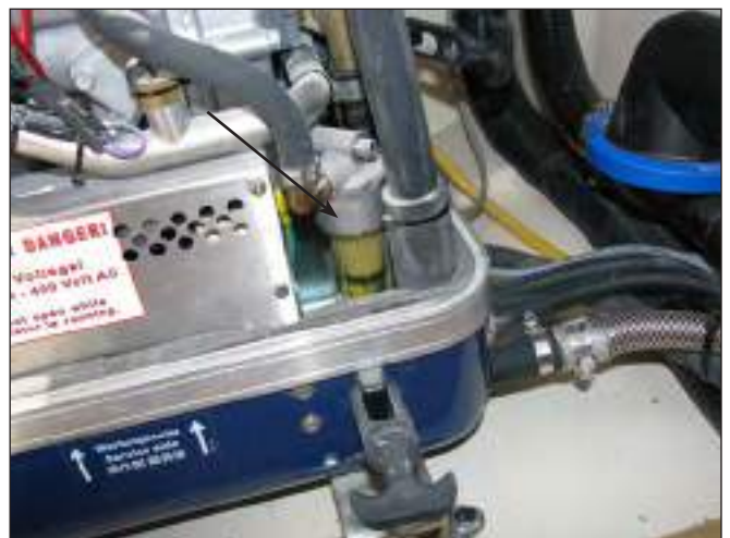
Typical Fuel Filter On the Generator
