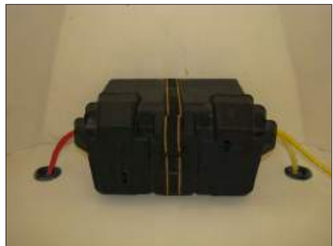
Optional Bow Thruster Battery In Below Deck Storage Compartment
