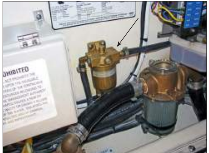
Typical Generator Fuel Filter
