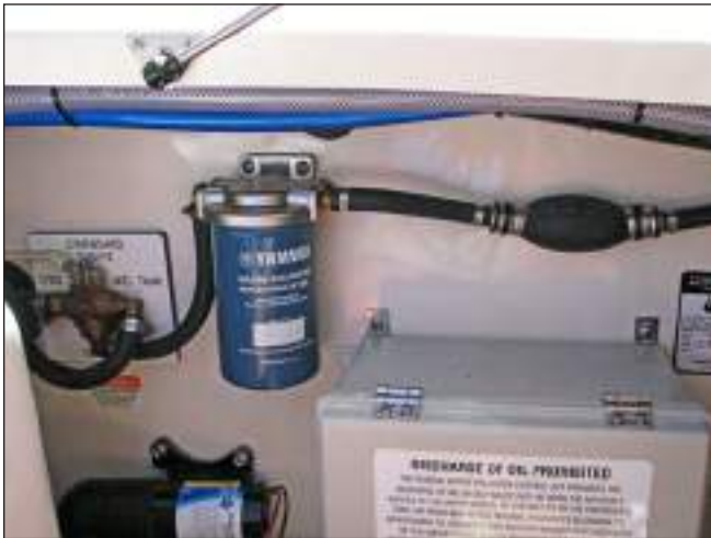
Triple Engine Fuel System - Stbd Engine Fuel Filter, Primer Bulbs & Fuel Selector Valve
