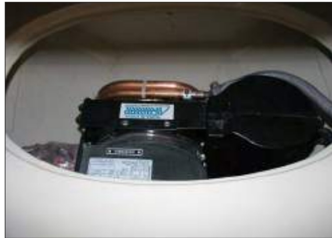
Air Conditioner Unit
