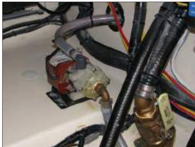
Air Conditioner Seawater Cooling Pump
