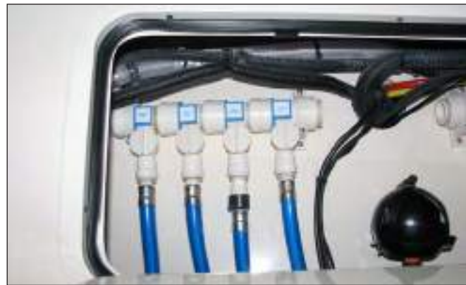
Cold Water Shutoff Valves Near Water Tank
