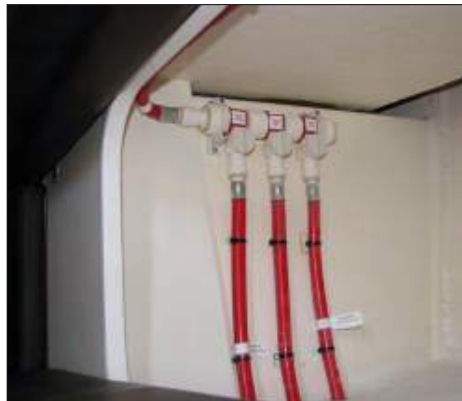
Hot Water Shutoff Valves Near Water Tank
