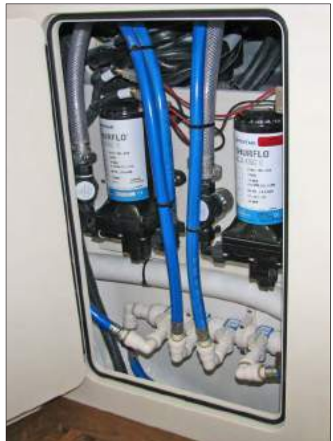
Typical Fresh Water Pump & Valve System
