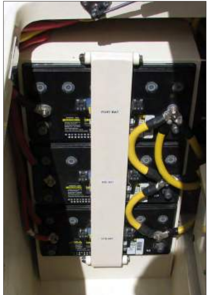
Typical Triple Engine Starting Batteries
