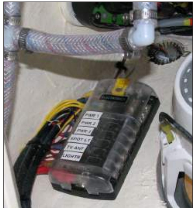
Typical Electronics Fuse Panel
