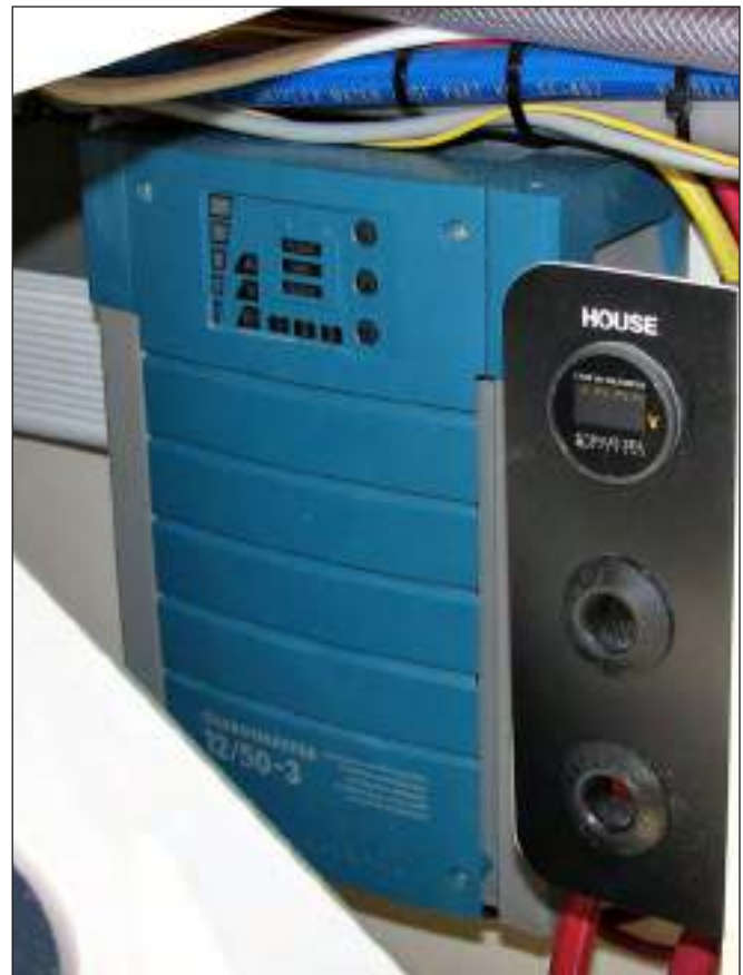
Typical Battery Charger & Volt Meter
