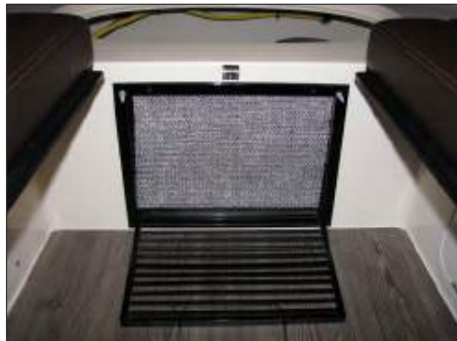
Air Conditioner Return Air Duct & Filter
