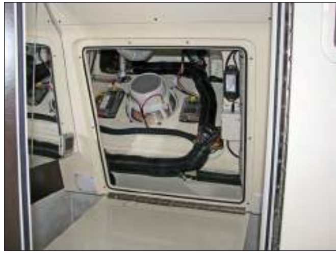
Upper Helm Access Panel Open & Helm Fuse Panels
