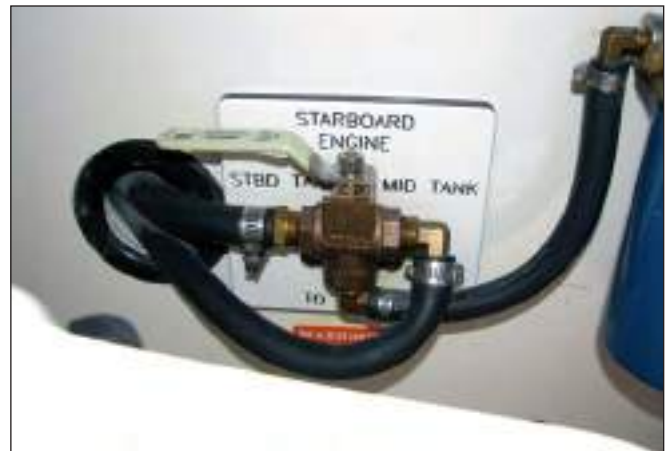
Triple Engine Fuel System - Stbd Engine Fuel Selector Valve
