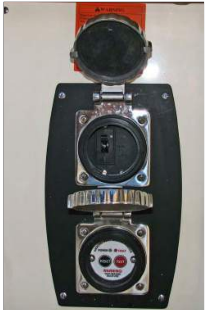
Shore Inlet Main Breaker & ELCI Panel In Cockpit
