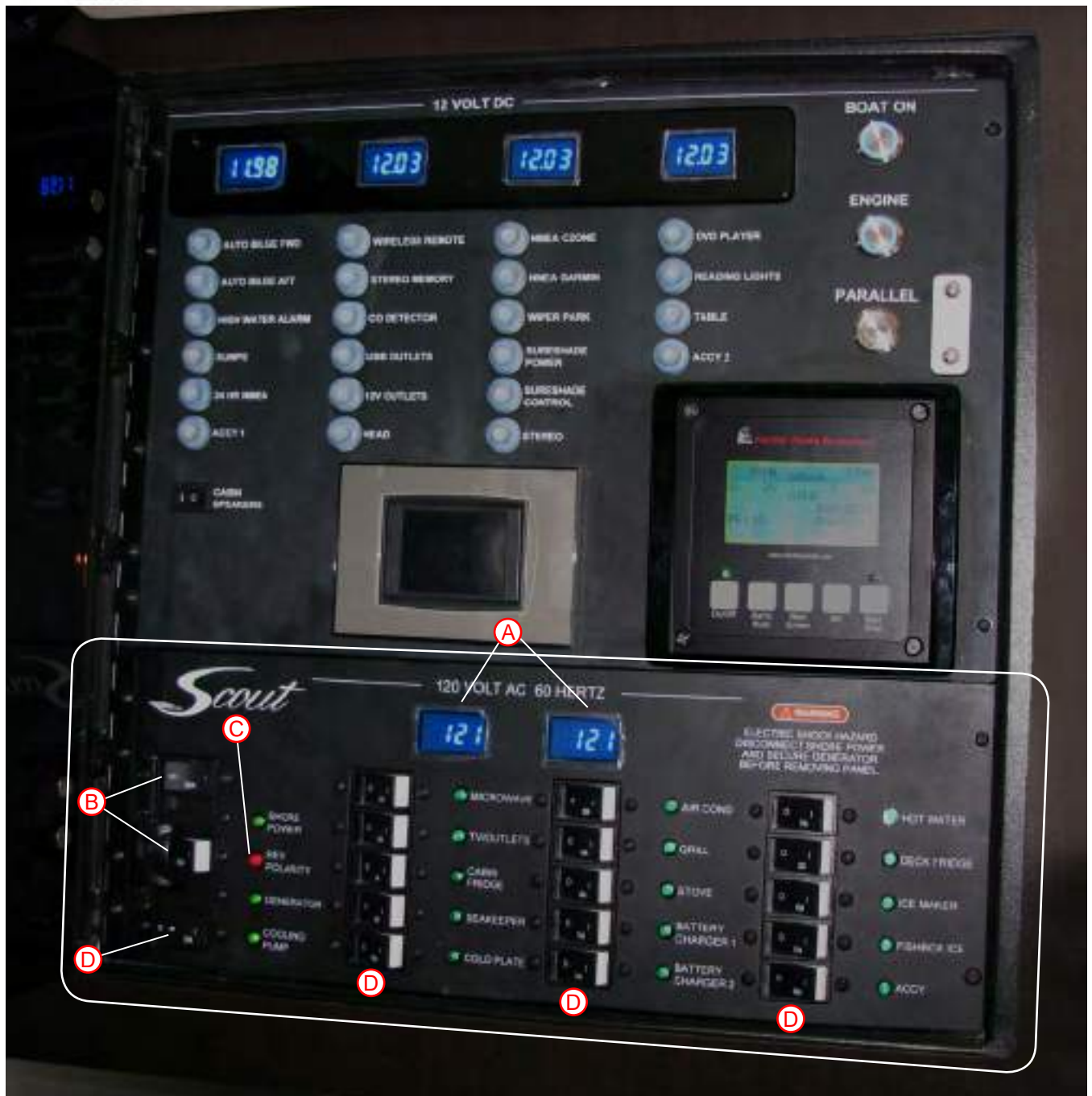
AC Main Distribution Panel
