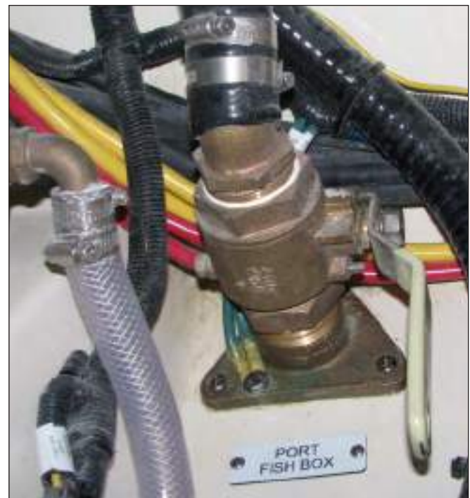
Thru-Hull Valve Bonding Wires & Connection
