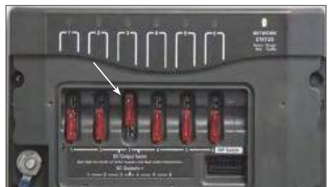
CZone Circuit 3 Fuse In Bypass Position
