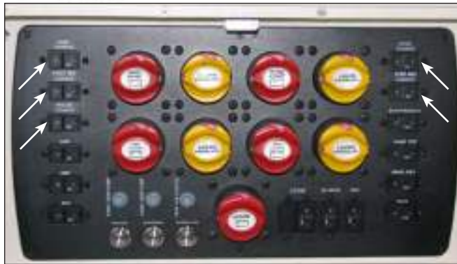
Quad Engine Battery/Charger Circuit Breakers
