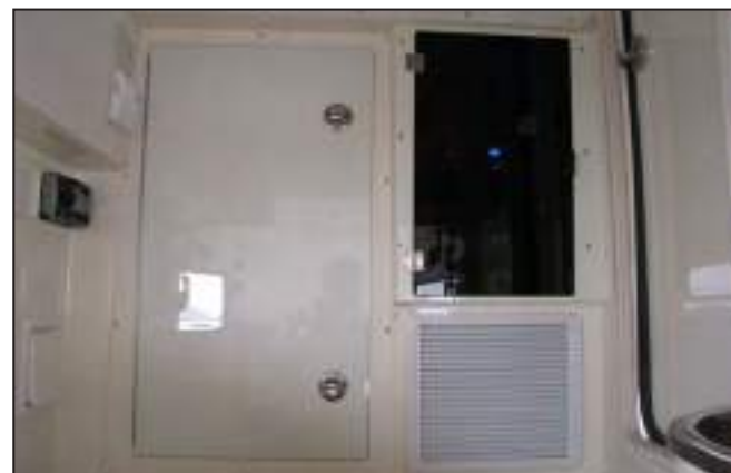
Cabin Breaker Panel and Helm Access Door
