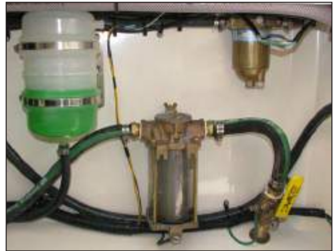
Primary Generator Diesel Fuel Filter, Coolant Recovery Tank, Sea Strainer and Intake Valve
