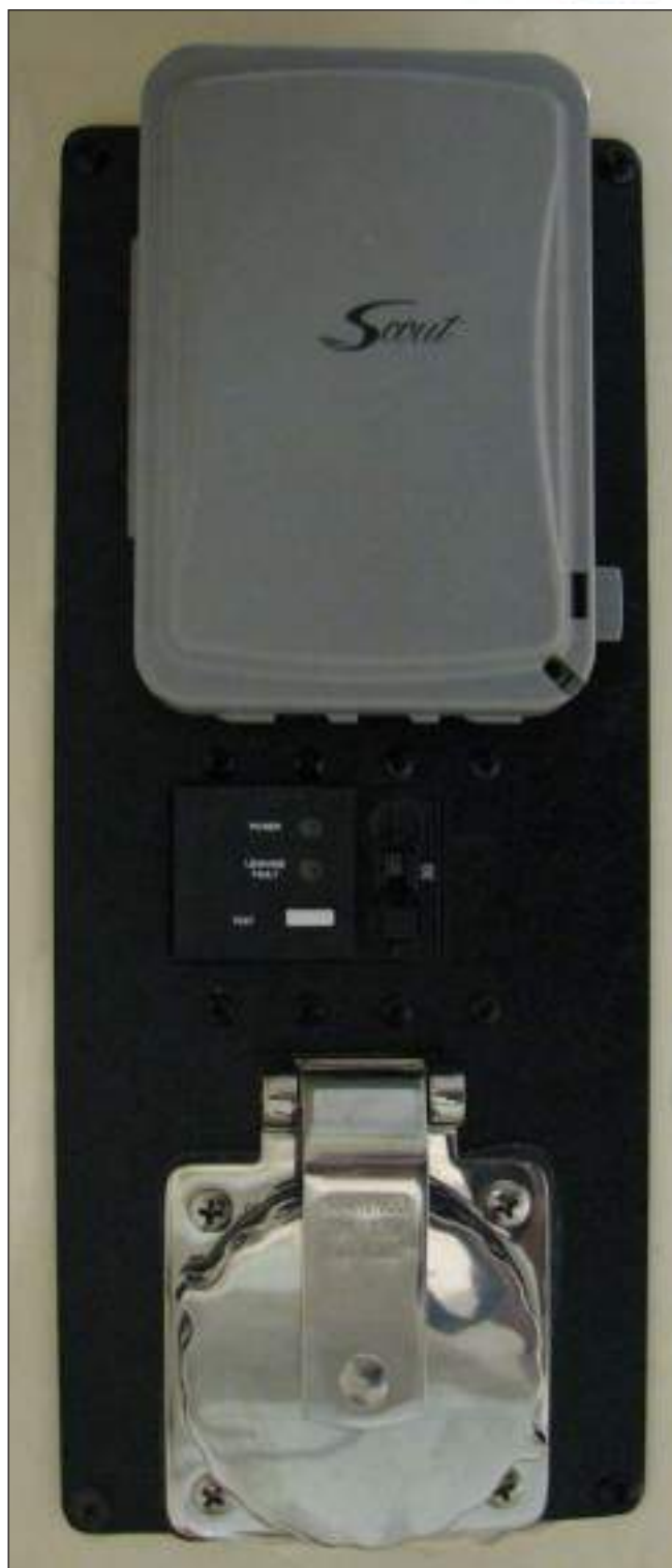
Boat AC Inlet, Main Circuit Breaker and ELCI Power Available Light and AC GFI Outlet
