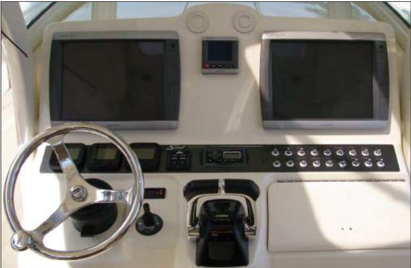
Helm Switch Panels, Bow Thruster Switch, Freezer Control Panel, and Trim Tab Switches
