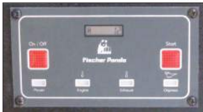
Typical Generator Control Panel
