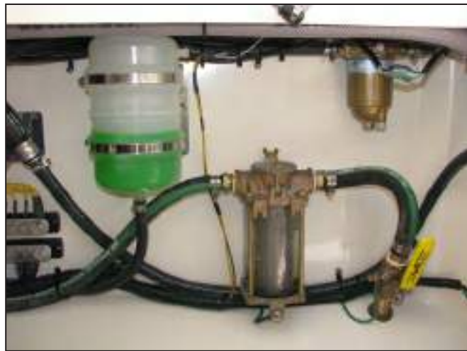
Generator Sea Strainer and Thru-Hull Valve
