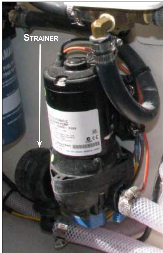
Raw Water Washdown Pump and Strainer
