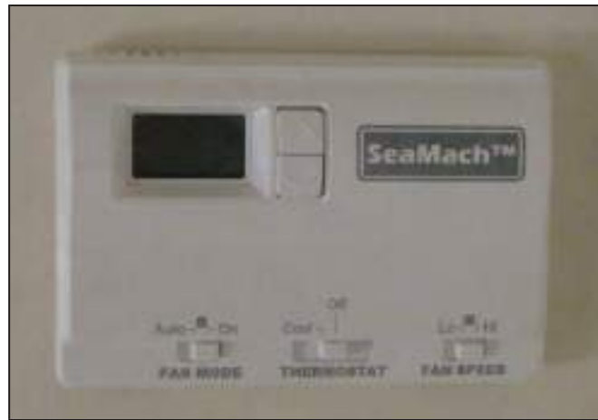
Cabin Air Conditioning Control Panel
