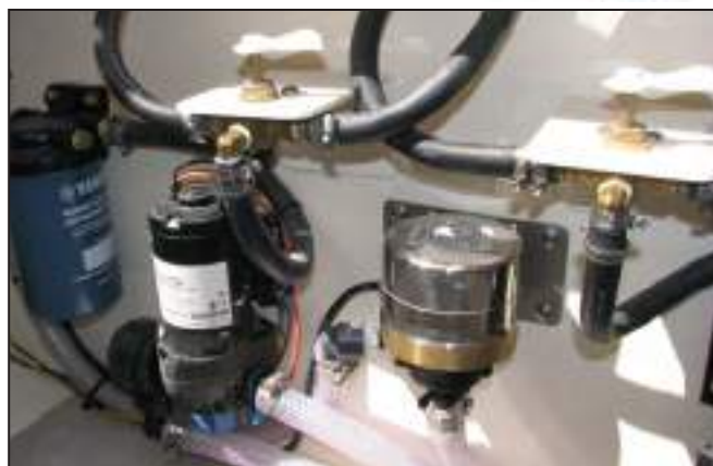
Raw Water Washdown and Air Conditioning/Freezer Circulating Pump
