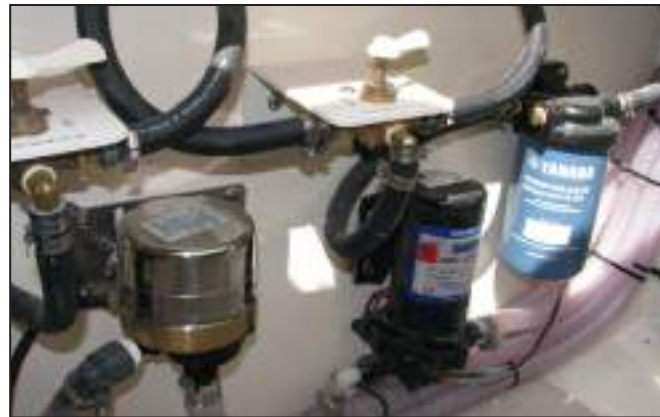
Starboard Engine Fuel Filter and Selector Valves in Stern Bilge
