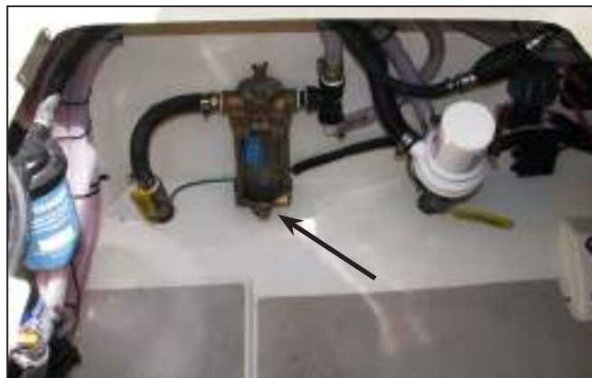
Seawater Intake Strainer for the Air Conditioning/Freezer Circulating and Raw Water Washdown Pumps
