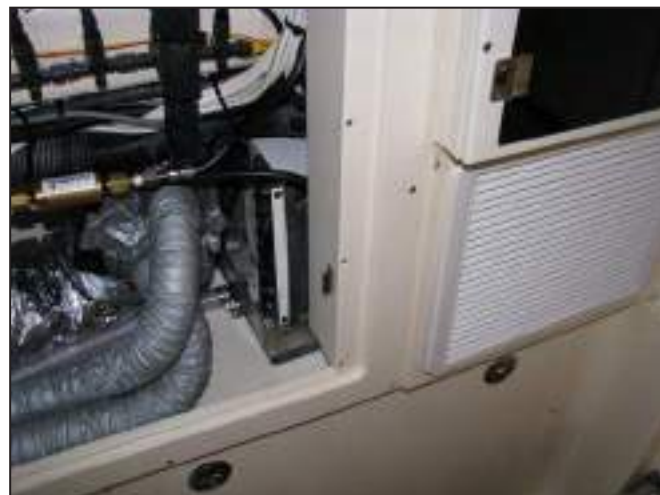
Cabin Air Conditioning Unit and Condensation Pan Drain
