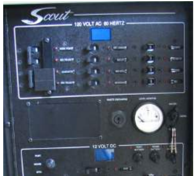
Waste Tank Gauge and Overboard Macerator Key Switch
