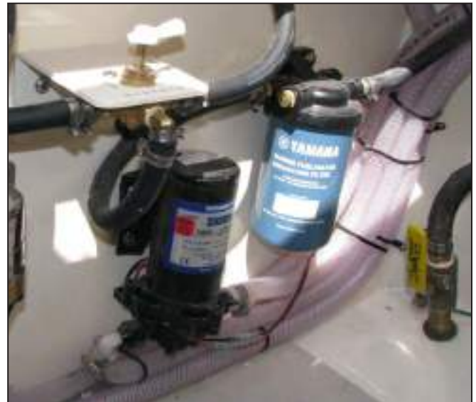
Fresh Water Pump in the Stern Systems Station
