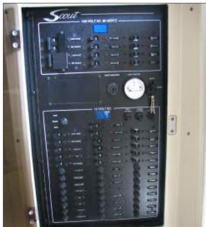
Cabin AC/DC Circuit Breaker Panel
