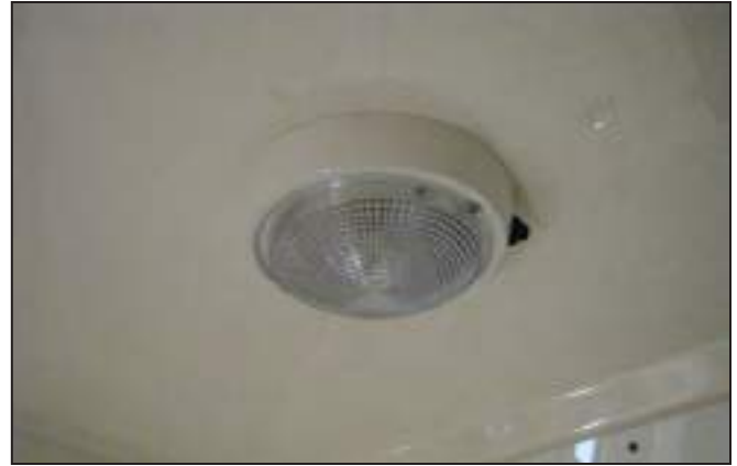
Overhead Light and Switch
