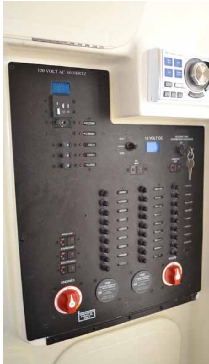
Battery Switches (red)
