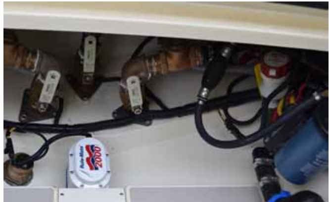
Bilge Pump and Baitwell Pumps
