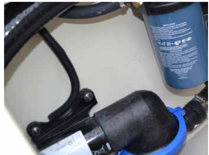
Overboard Discharge Pump in Stern Bilge
