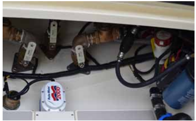
Baitwell and Bilge Pumps in Stern Bilge
