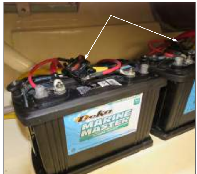
Engine Starting Battery Charging Wire Circuit Breakers
