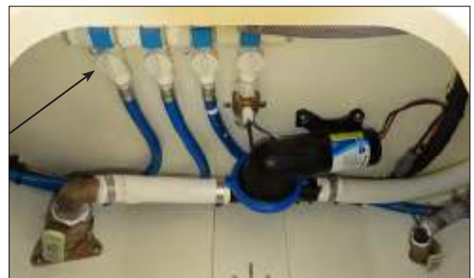
Fresh Water Manifold & Control Valves In Ski/Battery Storage Compartment
