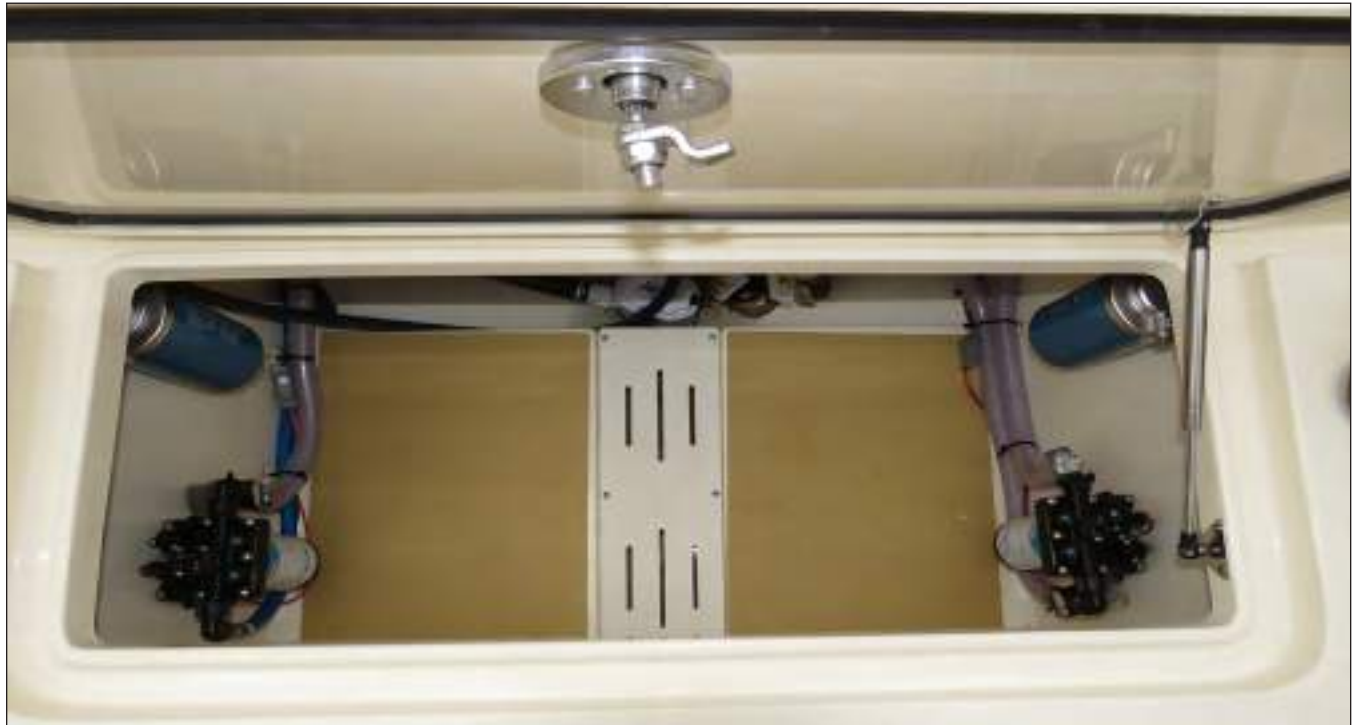
Aft Systems Compartment Showing Hatch Drain Rails & Bilge Pump
