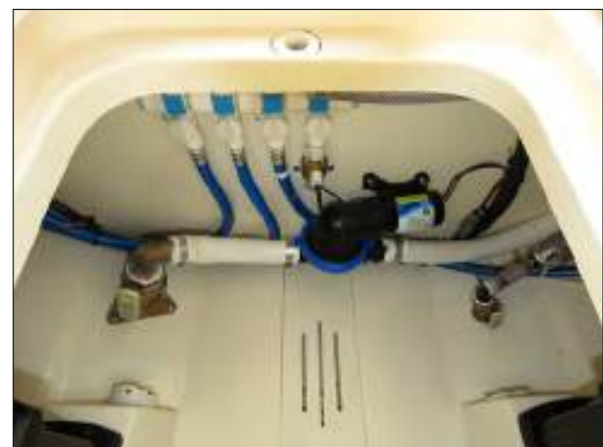
Freshwater System Valves & Optional Marine Toilet Valves In Ski/Battery Storage Compartment
