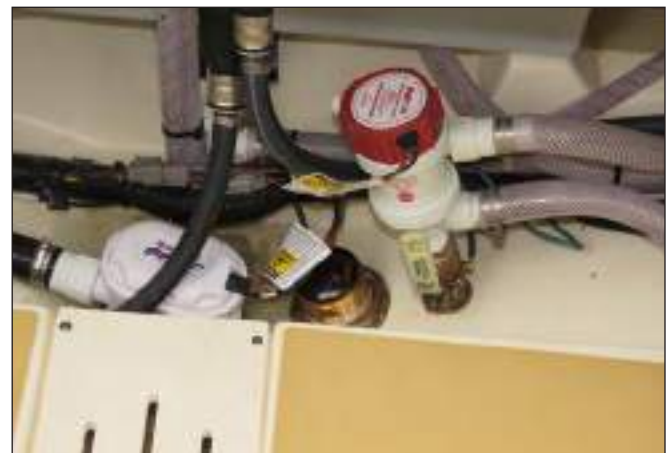
Baitwell Pump, Seacock Valve & Auxiliary Supply Fitting
