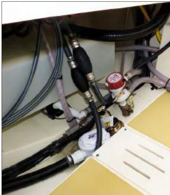
Typical Twin Engine Primer Bulbs In Aft Systems Compartment
