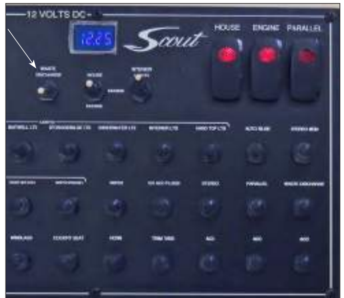
Waste Discharge Switch In DC Breaker Panel
