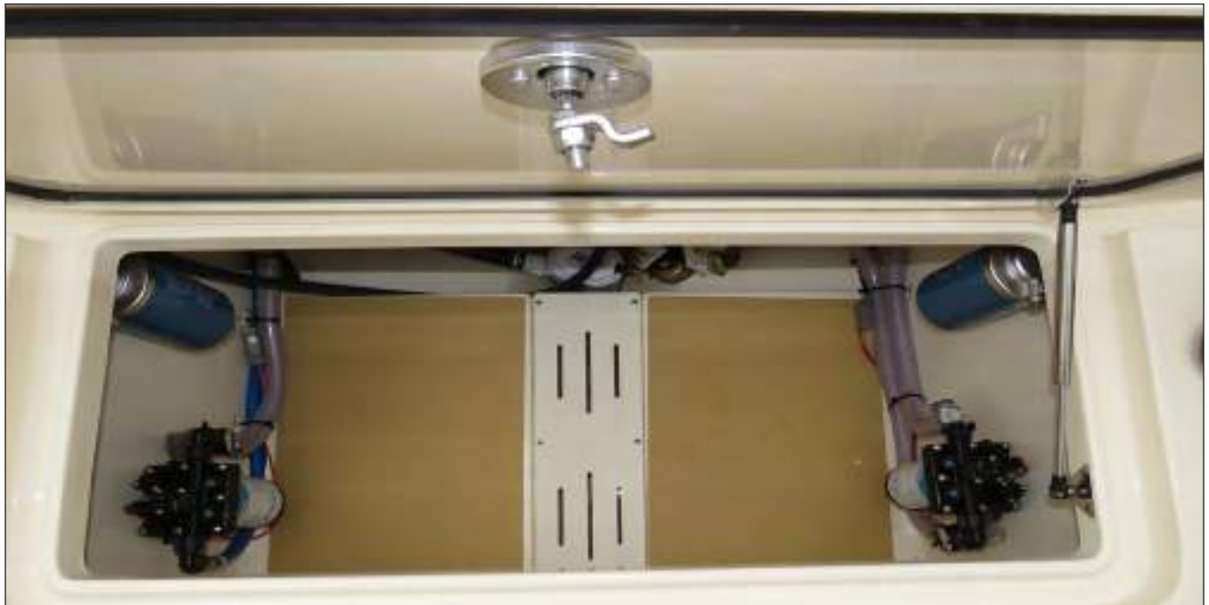
Aft Systems Compartment
