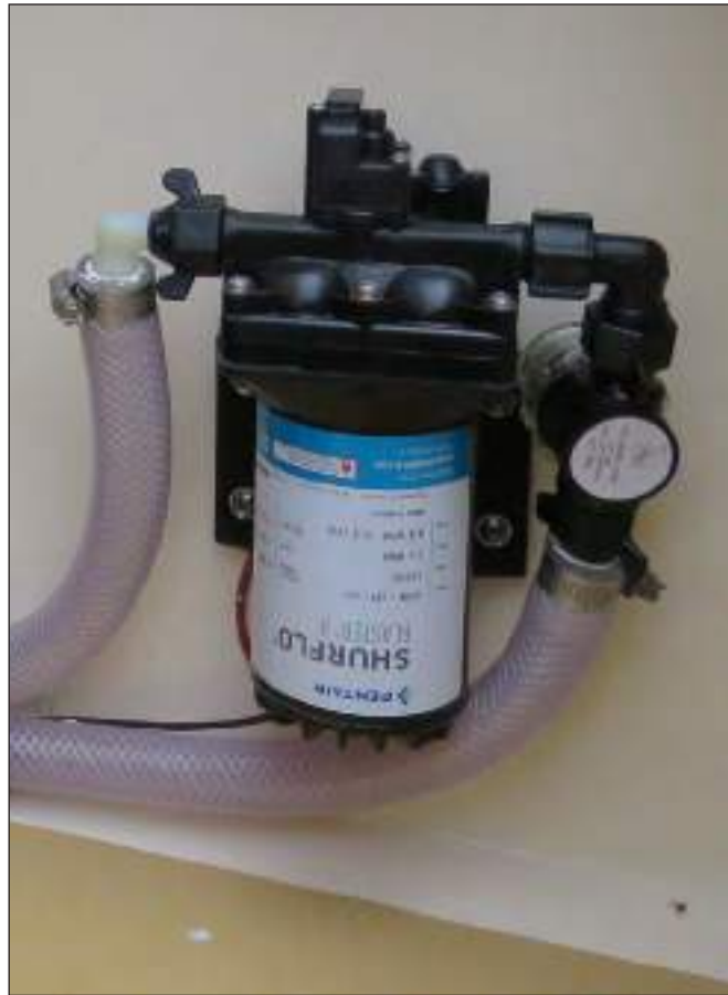
Raw Water Washdown Pump & Strainer
