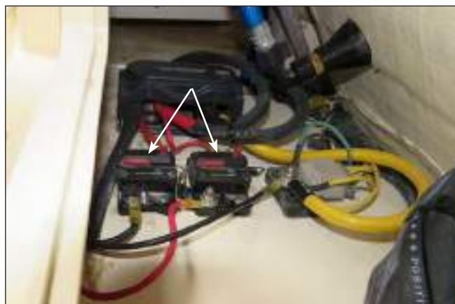
Typical Engine Charging Circuit & Power Steering Pump Circuit Breakers Located Behind The Aft Bench Seat.
