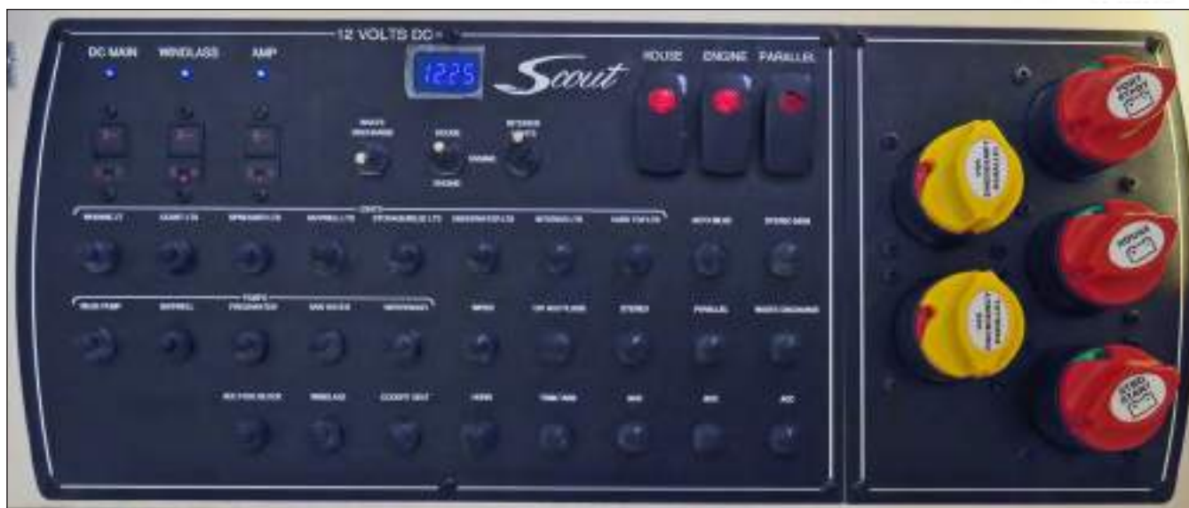
Twin Engine DC Breaker & Battery Switch Panels In Helm Storage Compartment
