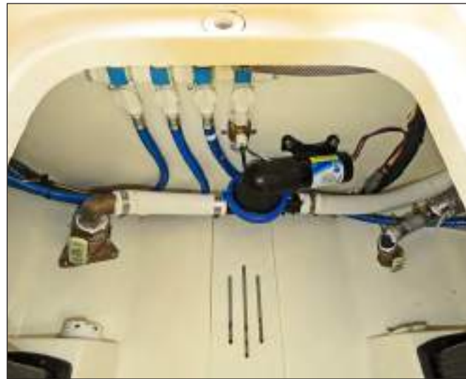
Marine Toilet Intake Valve, Overboard Discharge Valve & Waste Tank Pump
