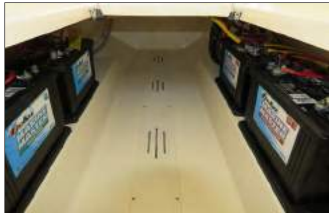
Typical Twin Engine Starting & House Batteries In Ski/ Battery Storage Compartment Below Cockpit Sole
