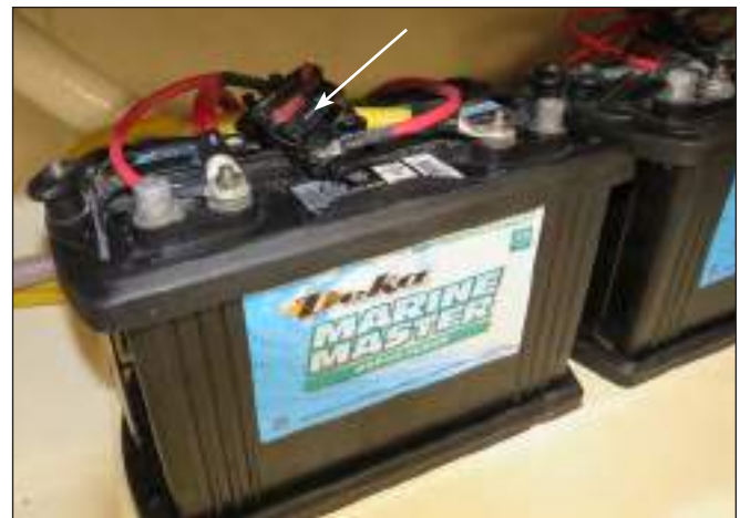
Battery Charger Circuit Breaker At Engine Starting Battery
