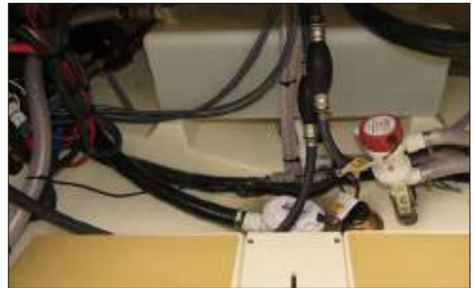
Fresh Water Tank In Aft Systems Compartment
