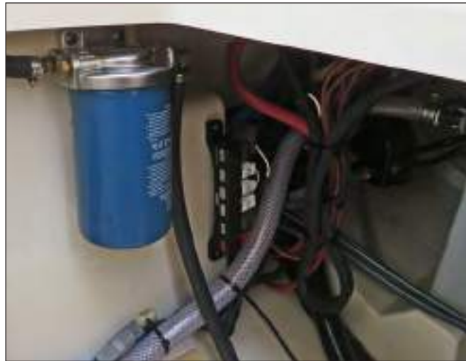
Engine Fuel Filter In Aft Systems Compartment
