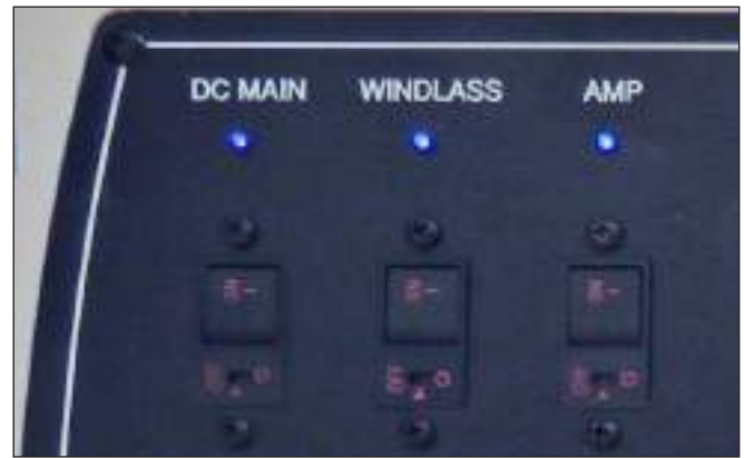
DC Panel Main Breakers
