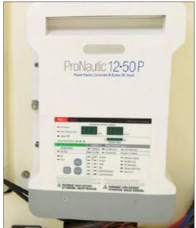
Typical Battery Charger
