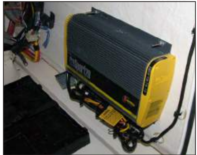
Typical Three Bank Battery Charger
