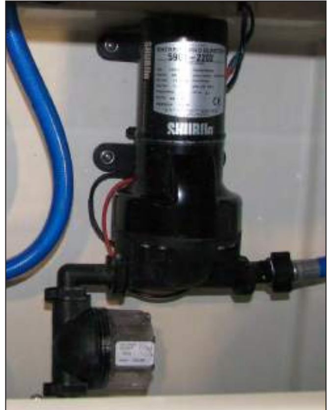
Typical Raw Water Supply Pump & Strainer
