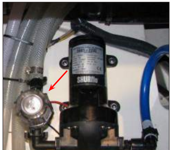
Typical Raw Water Pump Strainer
