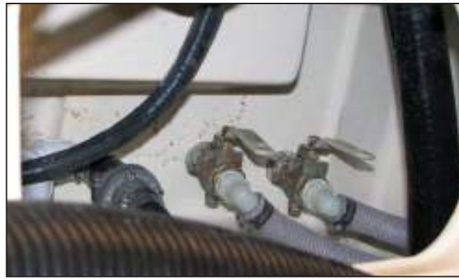
Typical Raw Water System Thru-Hull Valves
