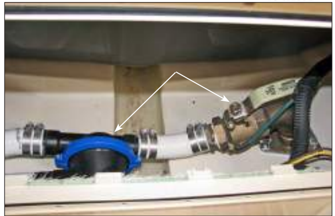
Typical Waste Discharge Pump & Thru-Hull Valve
