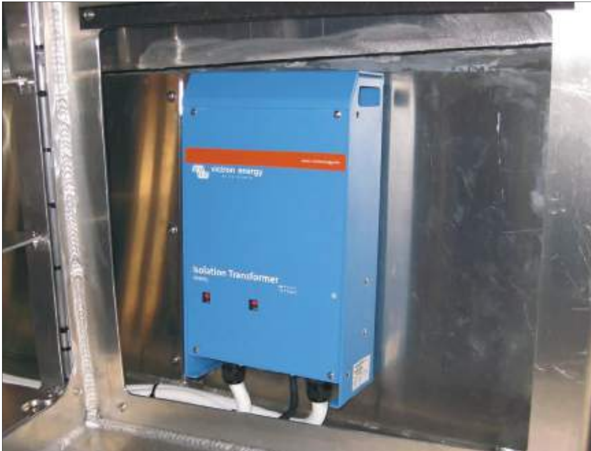
Figure 311-4a. Example Isolation Transformer
