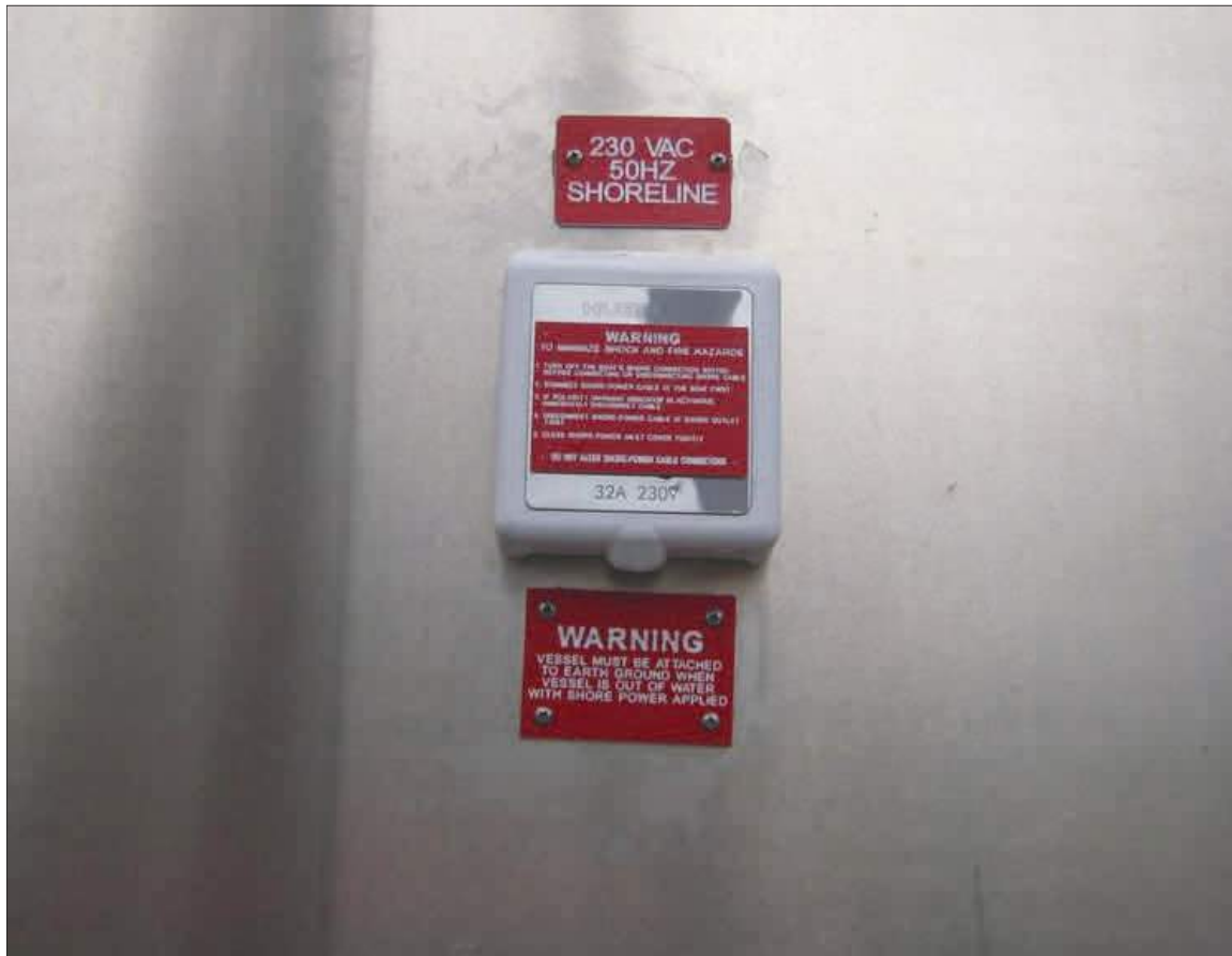
Figure 311-3a. Example Shore Power Connection
