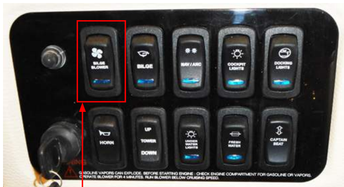
Bilge Blower Typical Switch Panel Shown
