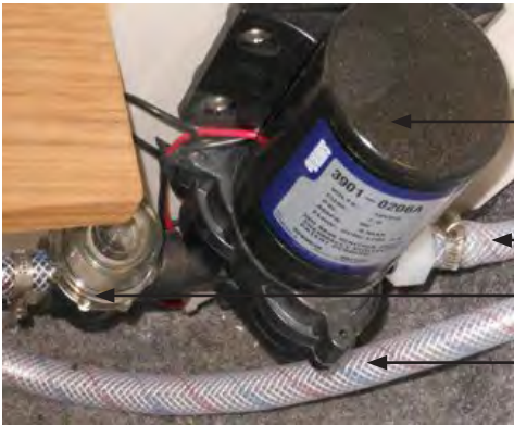
Typical Freshwater Pump
