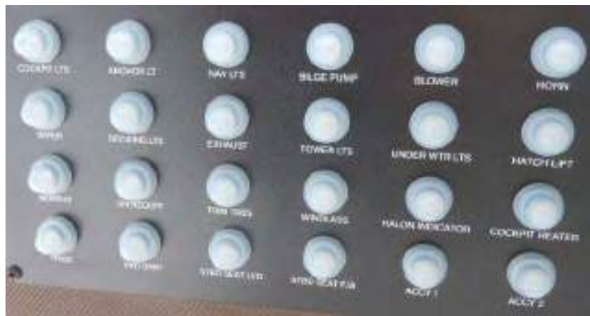
UNDER HELM BREAKER PANEL
