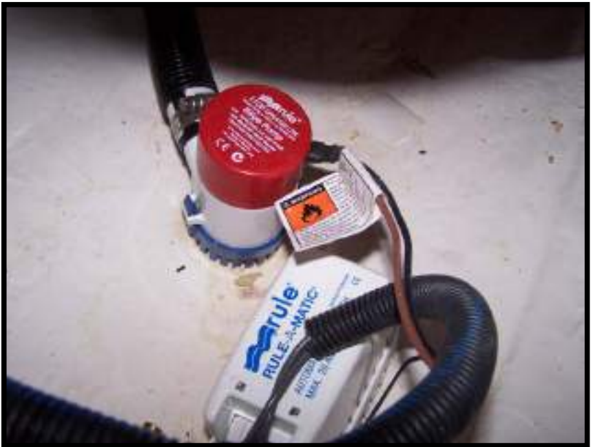
Typical Bilge Pump And Automatic Float Switch
