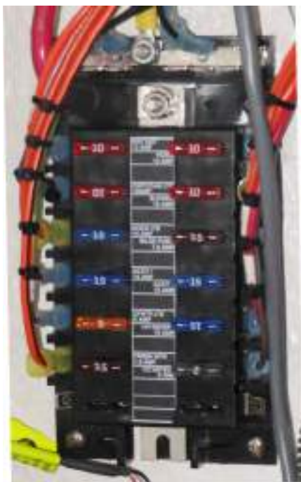
Typical Fuse Panel
