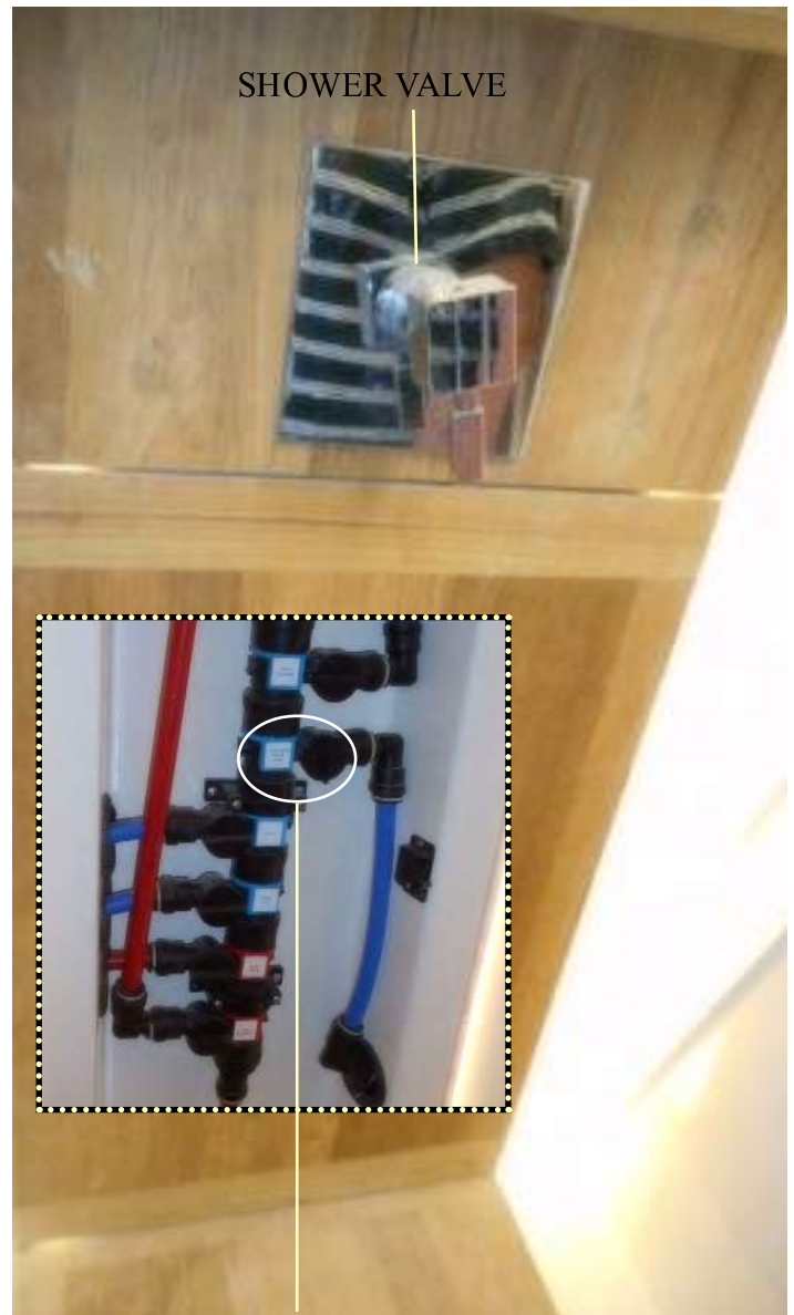
MASTER SHOWER TEAK LOCKER- FRESH WATER SYSTEM TANK SHUT-OFF VALVE INSIDE
