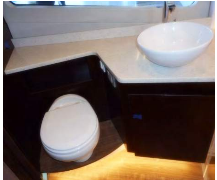
Typical Head w/ Vacuum Toilet & Vessel Sink
