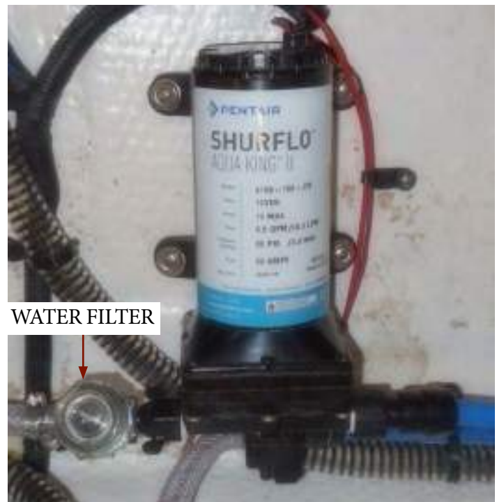
TYPICAL FRESH WATER PUMP
