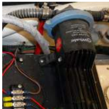
SHOWER PUMP (LOCATED IN ENGINE COMPARTMENT)
