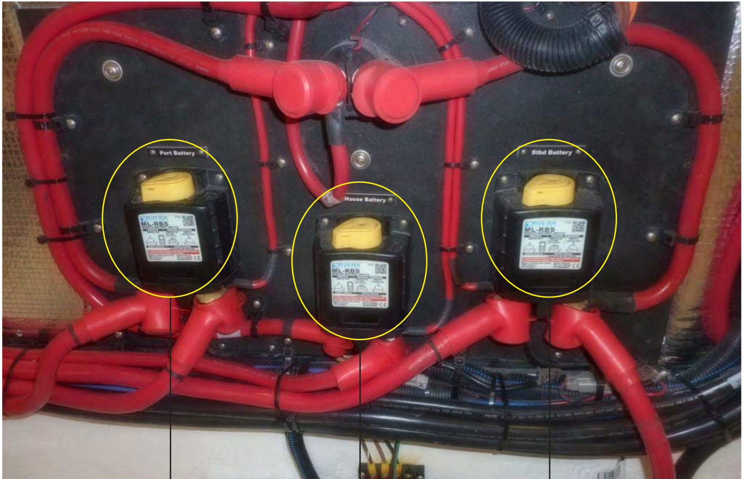
PORT REMOTE BATTERY SWITCH
