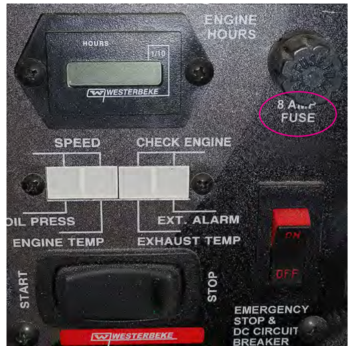
REMOTE GENERATOR PANEL SHOWING TOGGLE STYLE START/STOP SWITCH AND EMERGENCY STOP AND DC BREAKER
