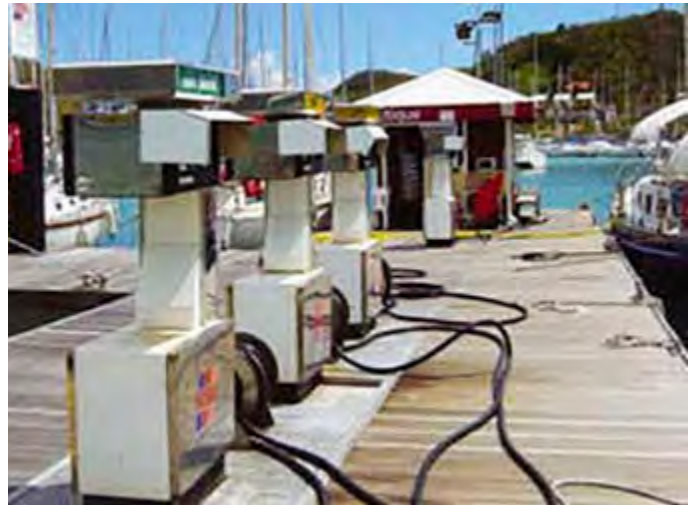
TYPICAL LARGE MARINA DIESEL FUEL DOCK
