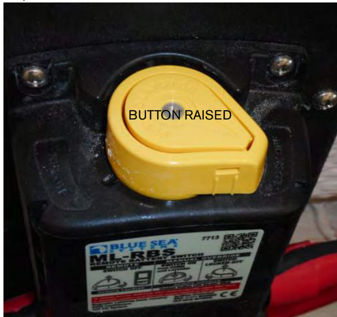
REMOTE BATTERY SWITCH LOCKED -OFF POSITION
