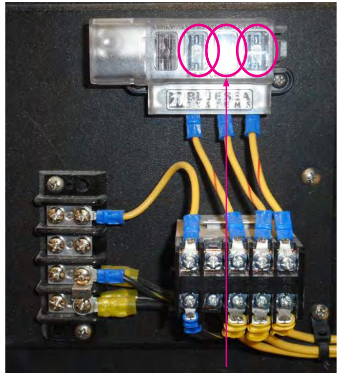
BLOWER RELAY PANEL SHOWING INDIVIDUAL FUSES WITH COVER
