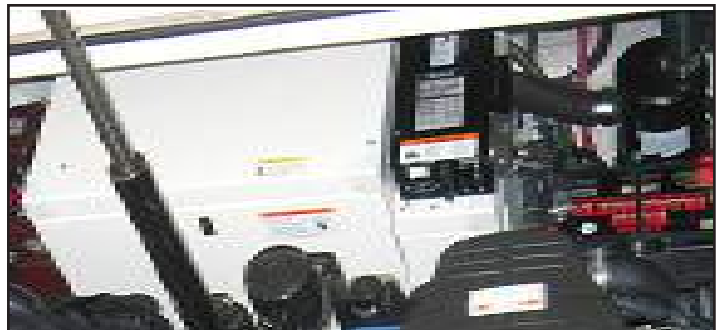
Typical Generator w/Sound Blanket
