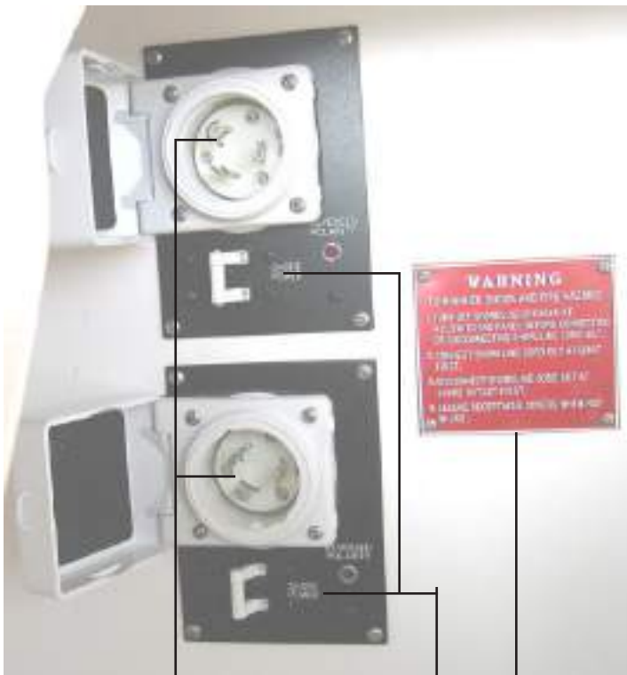
TYPICAL SHORE POWER INLETS
