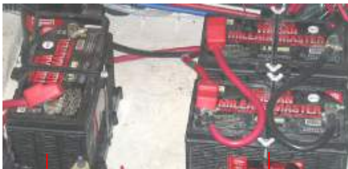
PORT ENGINE CRANKING BATTERY
