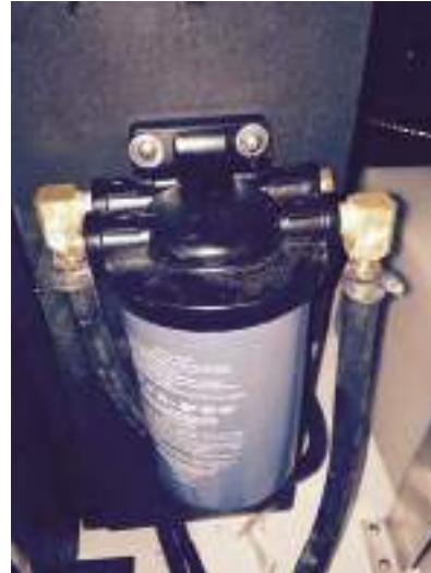
CHECKING IN-LINE WATER SEPARATOR FILTER
