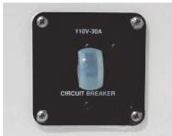
Shore Power Breaker
