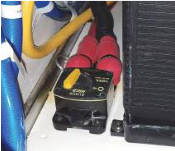
Main Battery Disconnect
