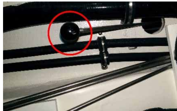
Deck drain ball valve levers
