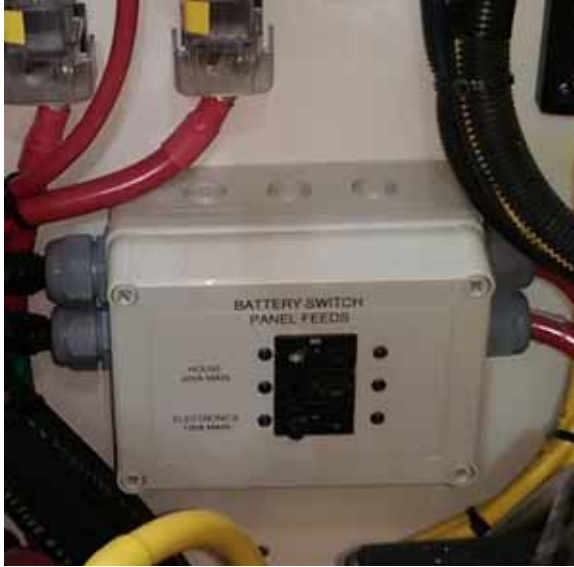
Main Electronics Battery Disconnect
