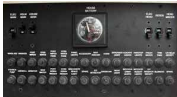
DC Main Distribution Panel (MDP)
