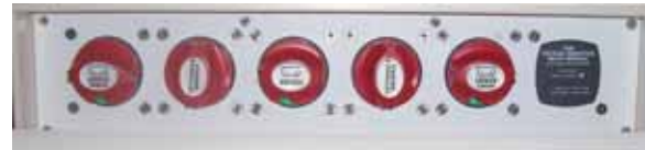
Battery Switch Panel
