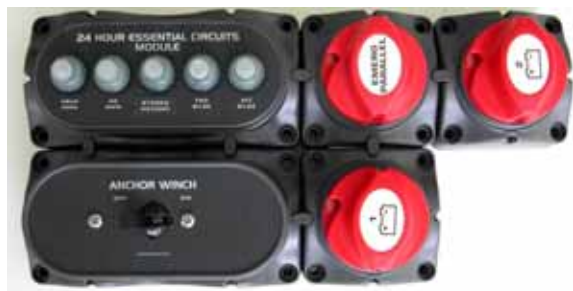
Battery Switches and Main Breakers Twin Engines (typical)
