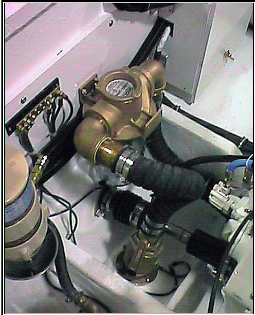
Figure 6-6: Engine Raw Water Intake
