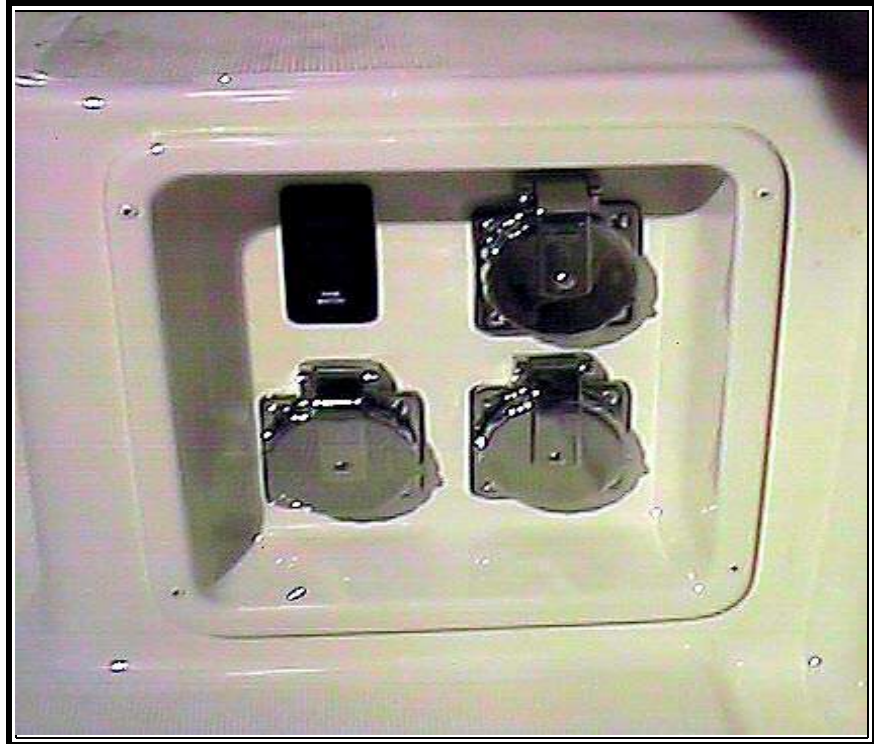
Figure 1-12: Shore Power Inlet
