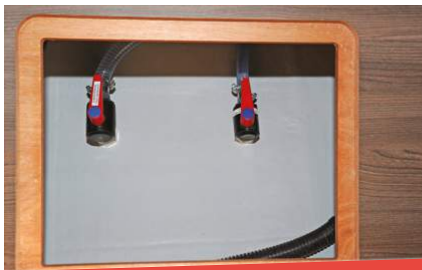
Seawater intake valve
