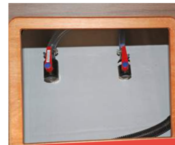
2 Seawater intake valve
