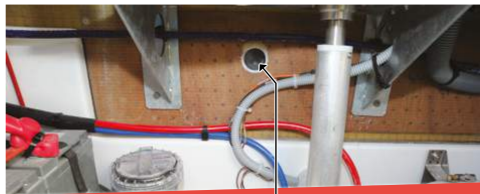
Fire extinguisher outlet starboard engine compartment
