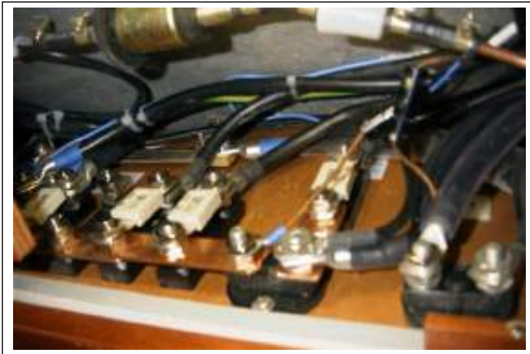
————— from left 1 = Technik Paneel 250Am 2= E-Winch BB 200Am ABB.: FUSES ————— 3= E.-Ankorwinch 100Am 4= Distribution Navi-Place 50 Am ABB.: MAIN FUSES 1= Anchor winch ————— 2 = General Consumption
