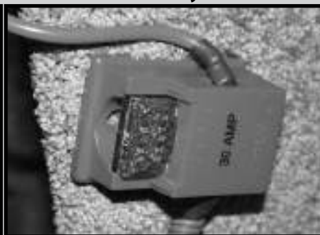
Fuse Panel - Battery Connection
