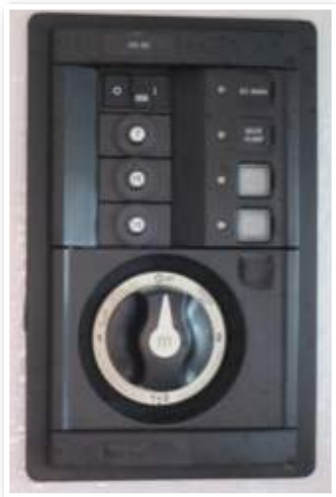
Battery Switch, Shown in the "Off" Position
