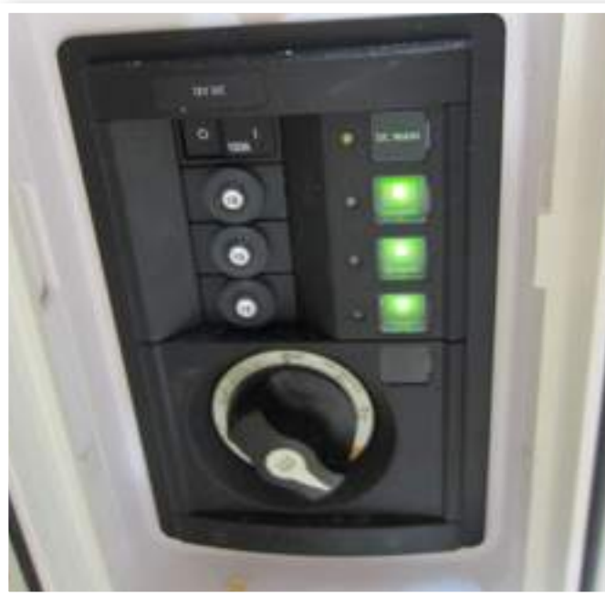
Battery Switch, Shown in the "Off" Position
