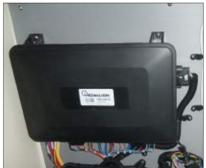
Power Management Module with Cover On
