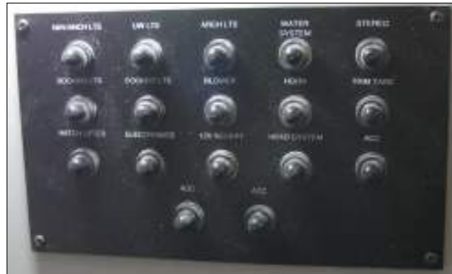
268SS Helm Accessory Circuit Breaker Panel
