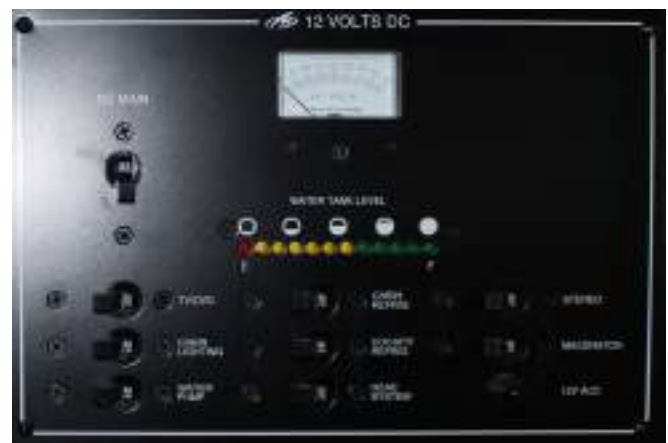
Cabin DC Electrical Panel
