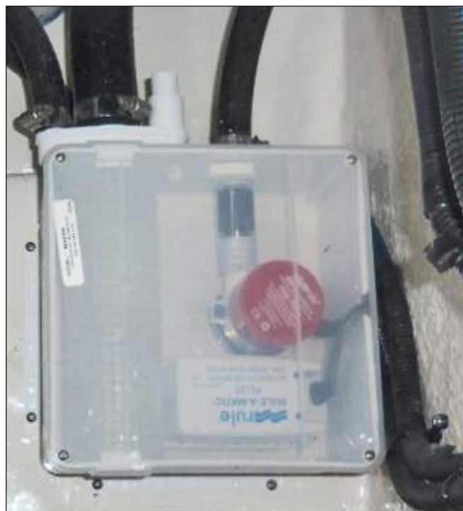
Sump Pump System
