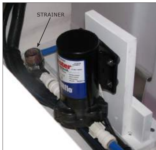
Typical Water Pump & Strainer
