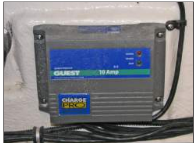
Typical Battery Charger
