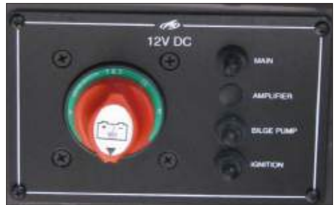
Battery Switch & Circuit Breaker Panel 214SS/218SS,234SS/238SS & 268SS
