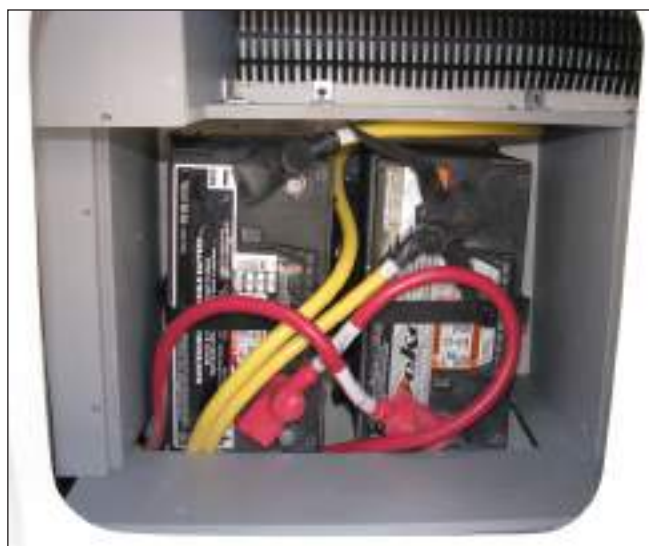
288SS Battery Installation Below Port Stern Seat
