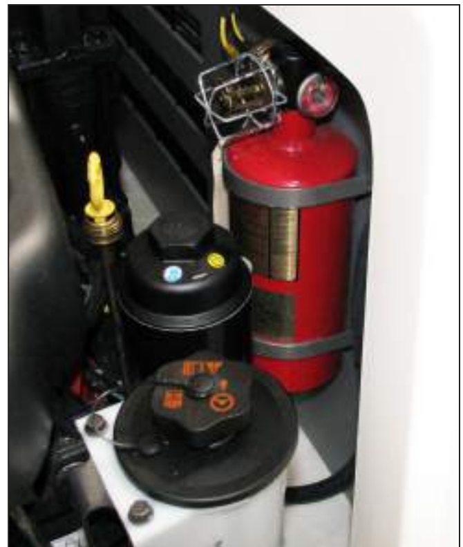
Automatic Fire Extinguishing System In The Engine Compartment
