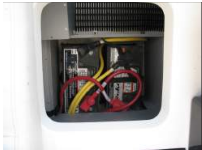
288SS Batteries In Aft Bench Seat Compartment
