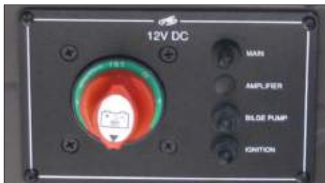
Typical 268SS Dual Battery Switch Panel
