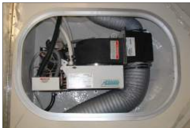
Typical 120-Volt Air Conditioner Below Berth
