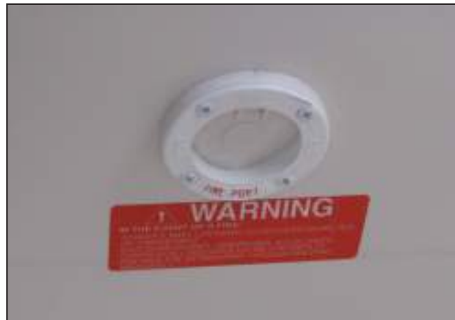
Typical Fire Port
