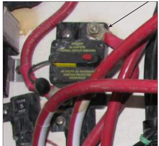
268SS Windlass Circuit Breaker Near Starboard Battery In Engine Compartment
