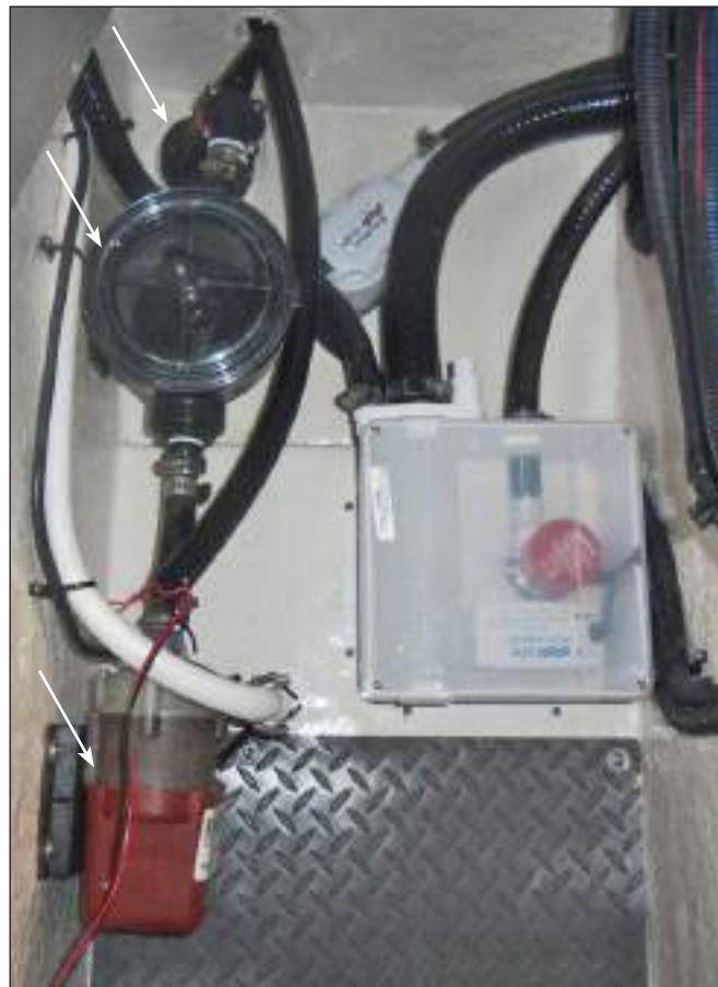
Air Conditioner Pump, Strainer & Thru-Hull Valve
