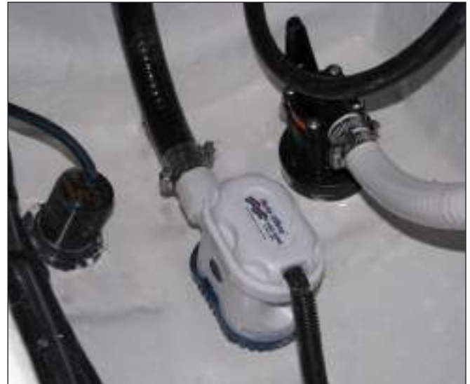
Typical Bilge Pump with Automatic Float Switch
