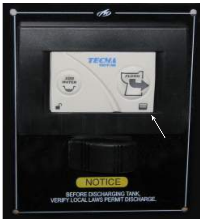
Head Compartment Toilet Control Panel
