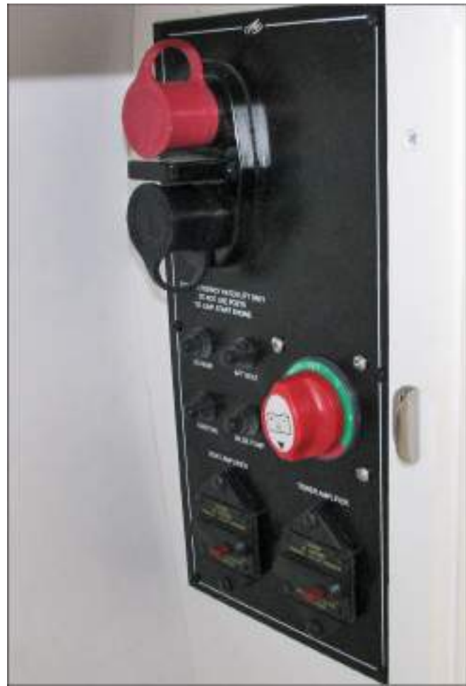
Dual Battery Switch Panel w/ Circuit Breakers, Engine Hatch Jumper Terminals & Sound System Amplifiers
