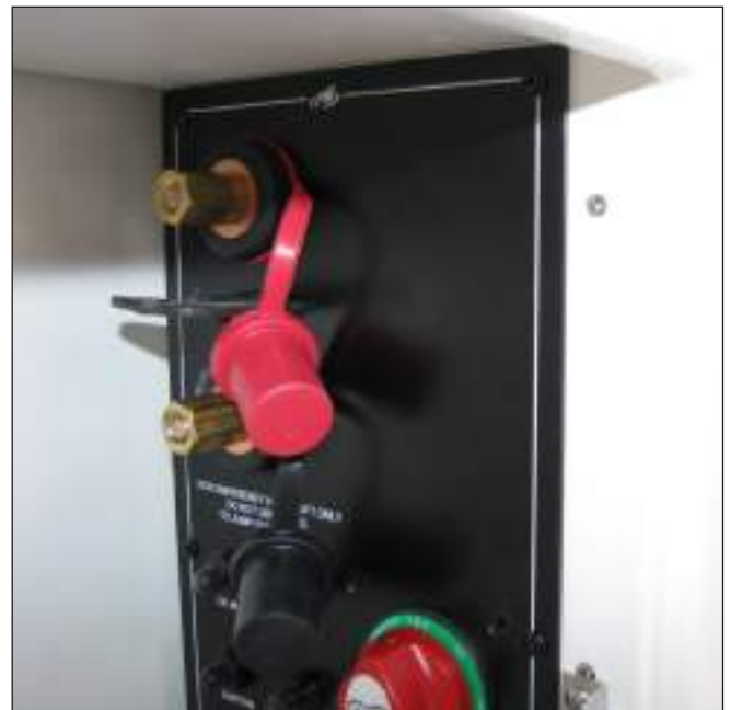
Access Hatch Jumper Terminal - Caps Removed
