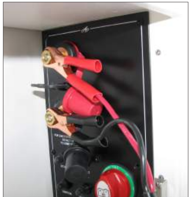
Jumper Harness Connected To Terminals
