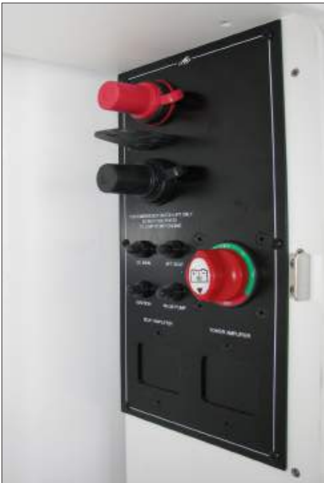
Dual Battery Switch Panel with Circuit Breakers & Engine Hatch Jumper Terminals
