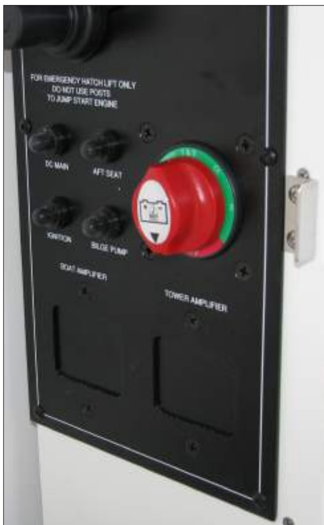
Battery Switch Panel Circuit Breakers
