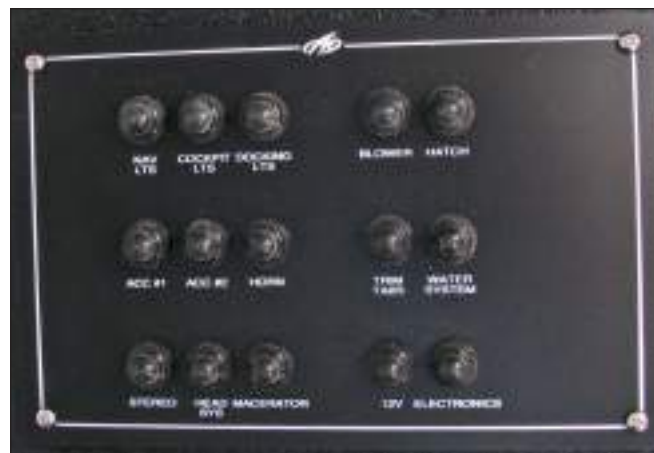
Main Helm Switch Circuit Breaker Panel
