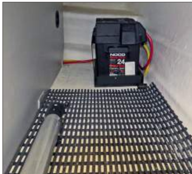
Battery Location In Storage Compartment
