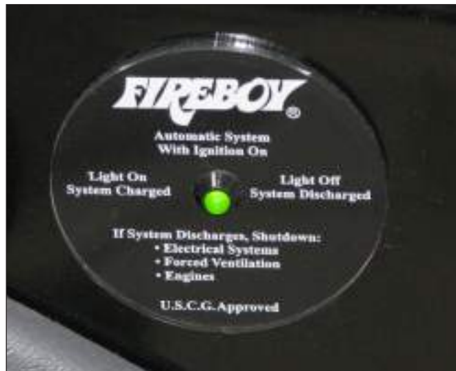
Typical Fire Extinguisher Panel In Helm
