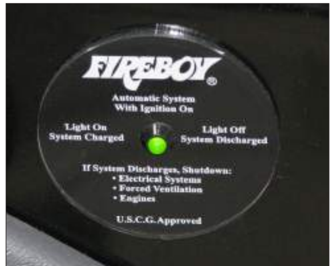
Typical Fire Extinguisher Panel In Helm
