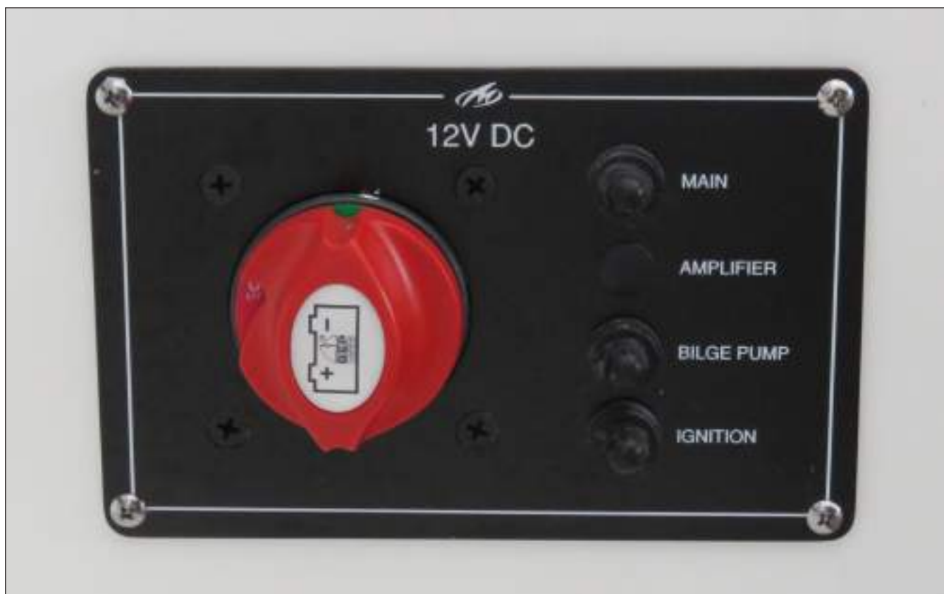
Battery Switch & Circuit Breakers
