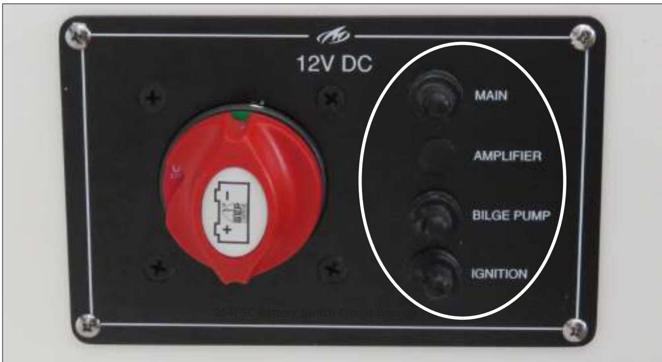
Battery Switch Panel & Circuit Breakers
