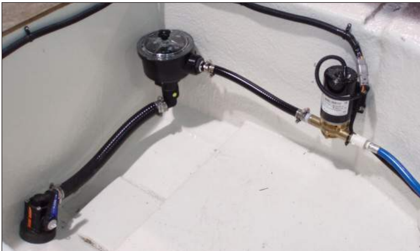
Ballast Pump Water System
