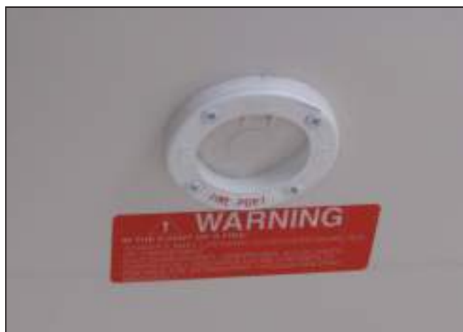
Typical Fire Port
