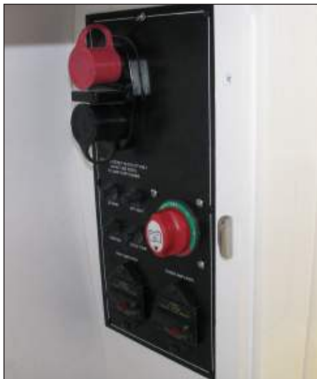
MSX Dual Battery Switch Panel w/ Circuit Breakers, Engine Hatch Jumper Terminals and Sound System Amplifiers
