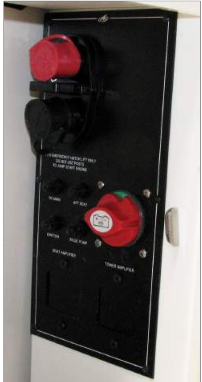
M4 Single Battery Switch Panel with Circuit Breakers and Engine Hatch Battery Jumper Terminals
