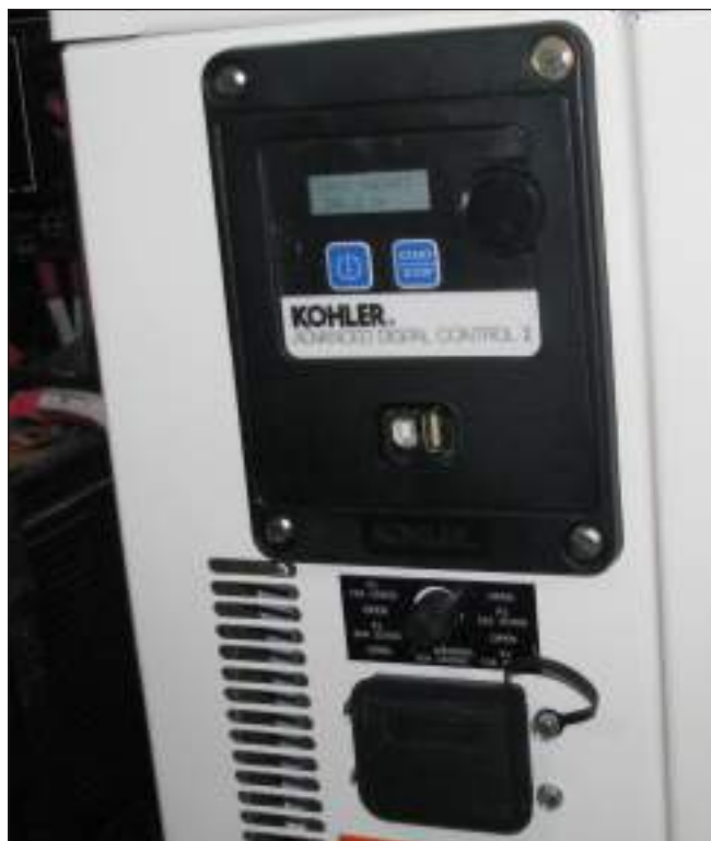
Typical Generator Control Panel
