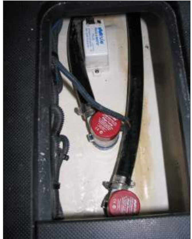
315SY Aft Bilge Pump, Emergency Bilge Pump & Aft Pump Automatic Switch In The Stern Bilge Between The Engines
