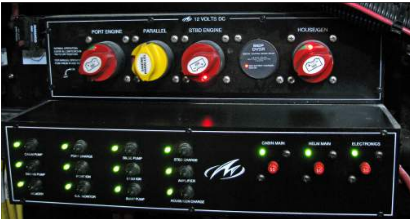
315SY Battery Switches & Battery Switch Circuit Breaker Panel
