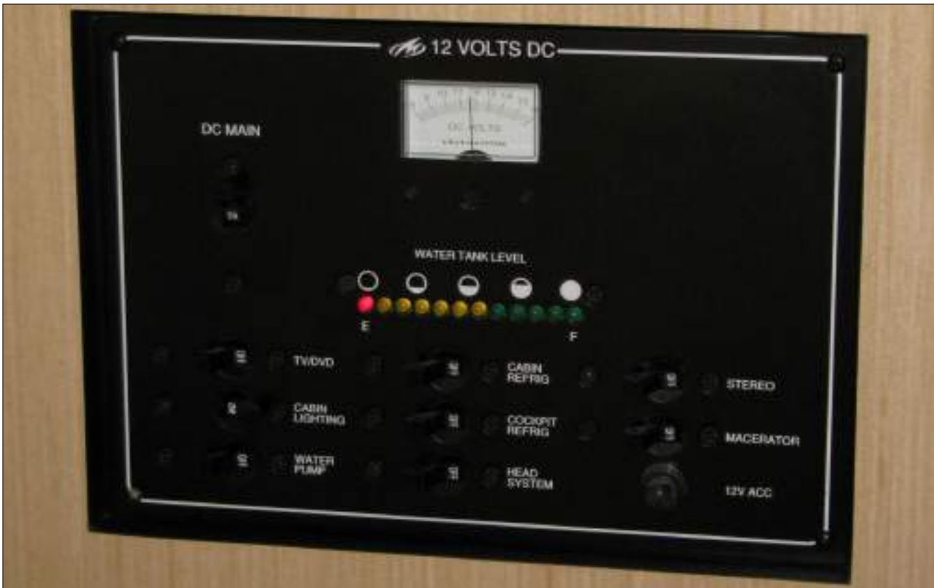
275/295SY Cabin DC Circuit Breaker Panel
