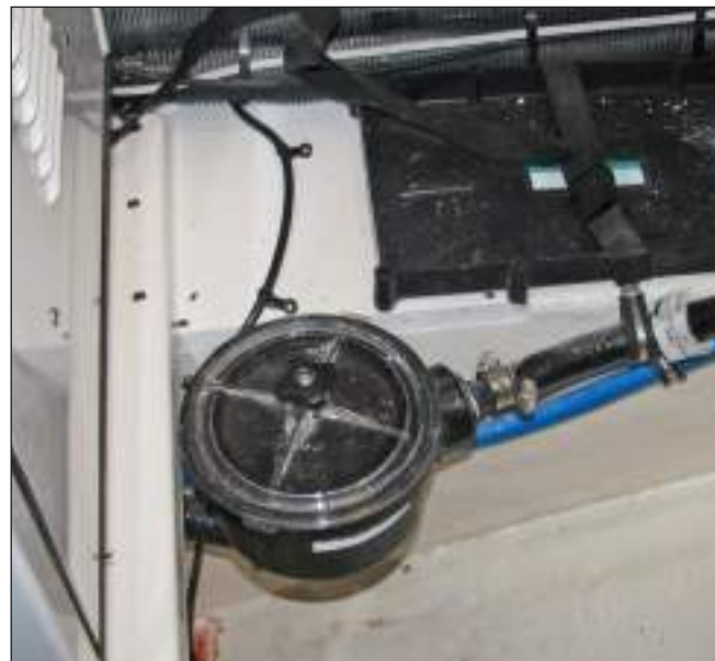
Air Conditioner Pump & Strainer
