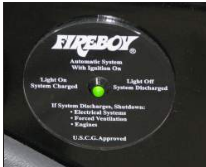
Fire Extinguisher Panel In Helm
