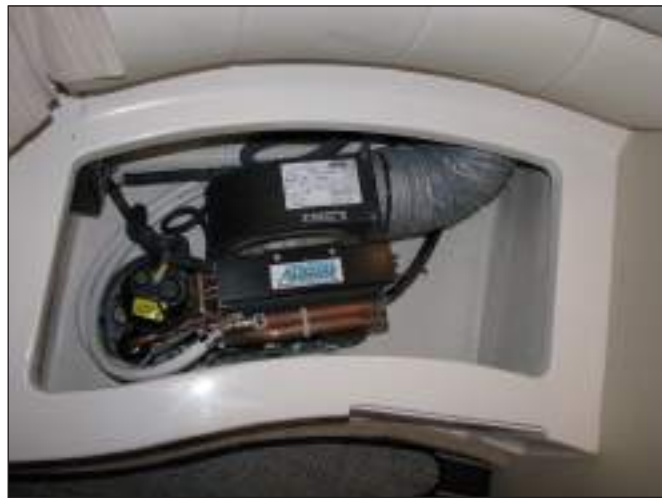
315SY Air Conditioner In Lounge Seat Storage Compartment
