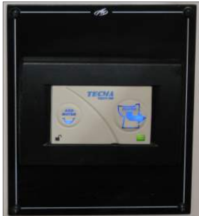
Tecma Toilet Control Panel & Overboard Macerator Discharge Switch
