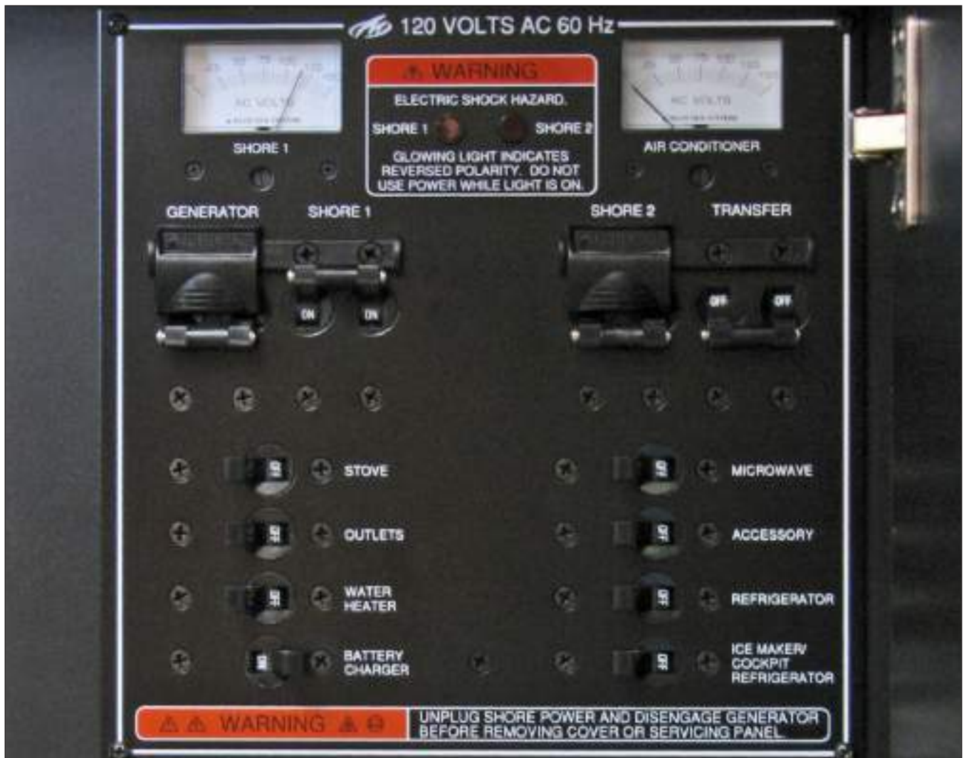
315SY 120 Volt AC Circuit Breaker Panel With Optional Generator & Air Conditioning
