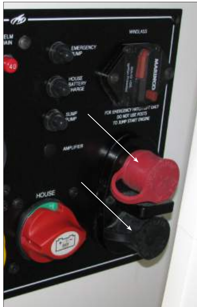
Battery Switch Jumper Terminals
