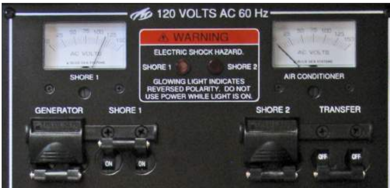
Typical 315SY 120 Volt AC Main Breaker Sliding Covers & Reverse Polarity Lights
