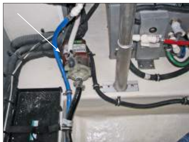
Typical Air Conditioning Pump In Engine Compartment
