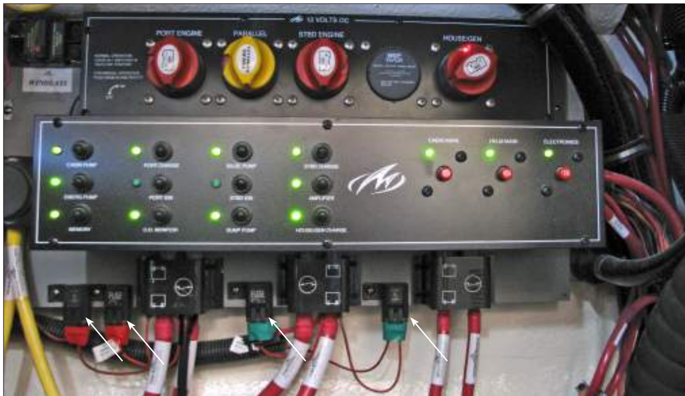
Typical 315SY Battery Switch Panel & Mercruiser Fuses
