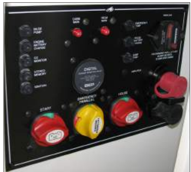
275/295SY Battery Switches & Battery Switch Circuit Breaker Panel
