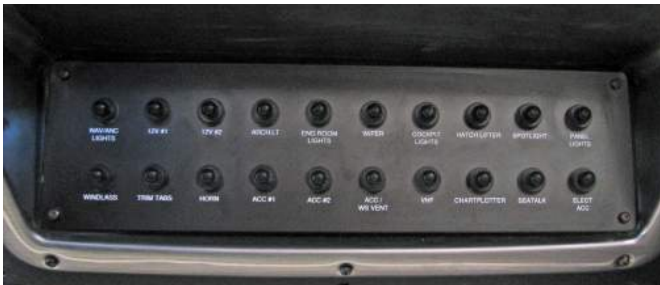
315SY Helm Circuit Breaker Panel
