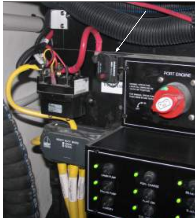
Windlass Main Circuit Breaker
