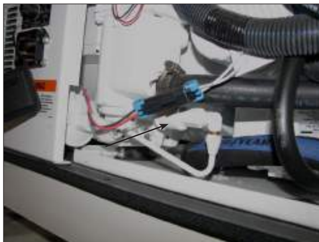
Typical Generator Fuel Filter
