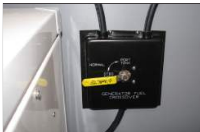
315SY Generator Fuel Tank Selector Valve Starboard Fuel Tank Selected
