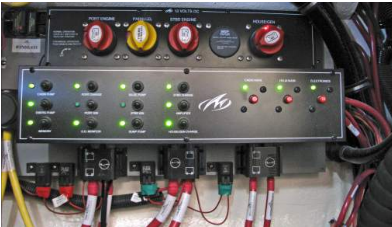
Battery Switch Panel, Battery & Parallel Switches, Main Circuit Breakers & Continuous Duty Circuit Breakers
