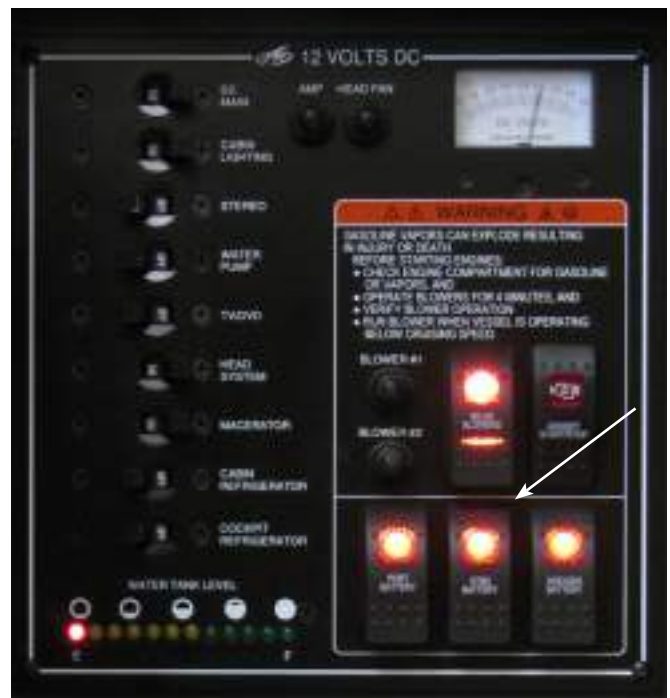
Remote Battery Switches in Cabin DC Panel
