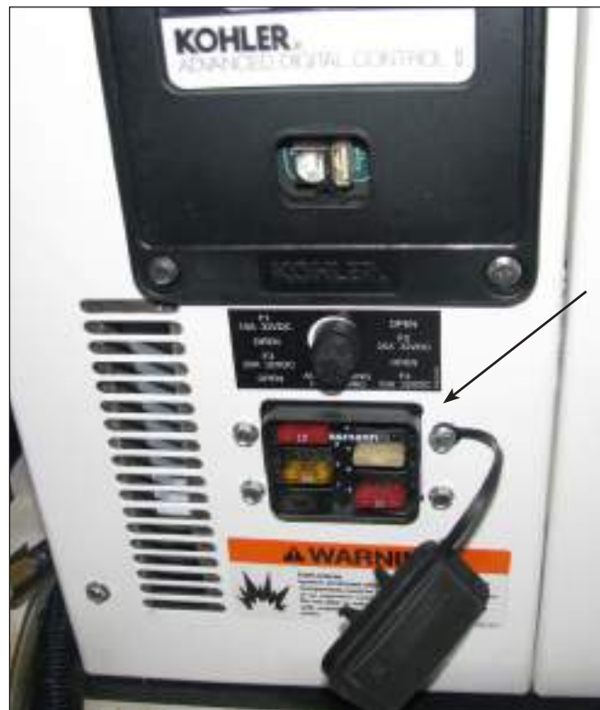
Typical Generator DC Circuit Fuse Panel
