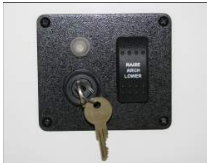
Arch Key Activated Switch & Circuit Breaker Panel
