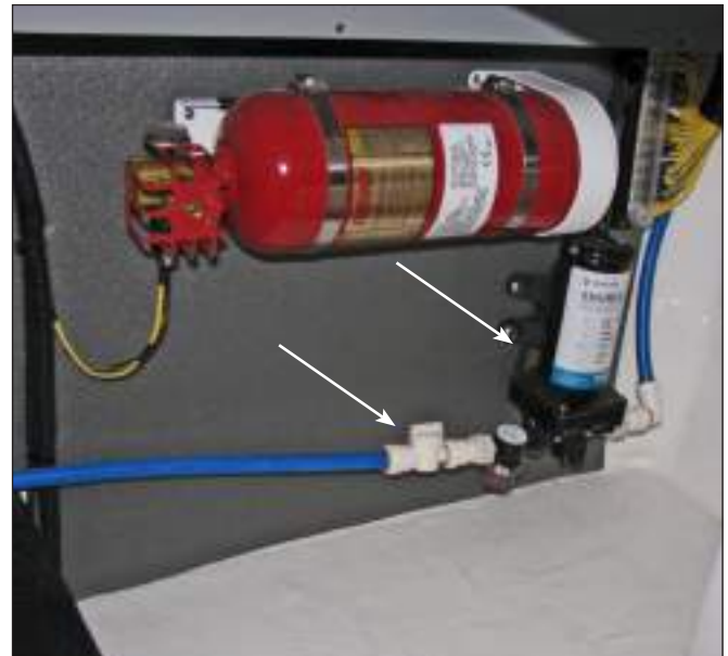
275/295SY Fresh Water Pump & Shutoff Valve
