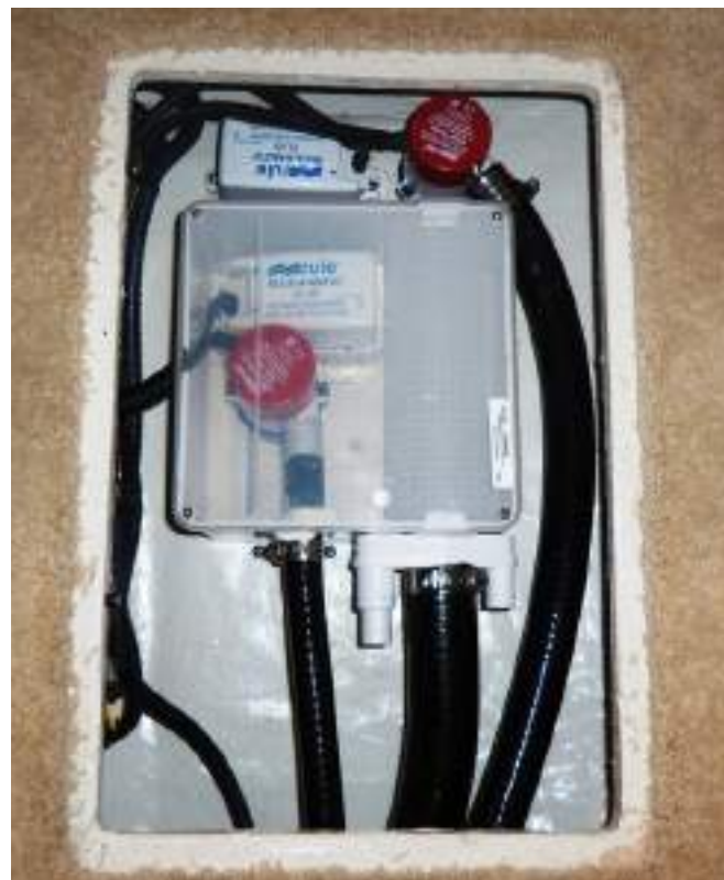
Forward Bilge Pump & Automatic Switch
