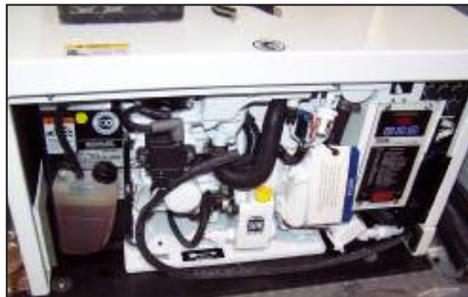
Typical Diesel Generator and Onboard Control Panel with Circuit Breakers
