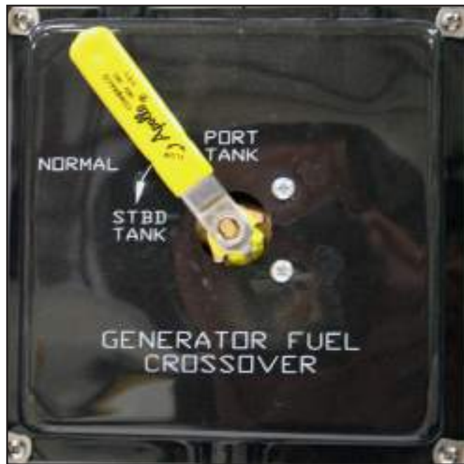
Generator Fuel Crossover Valve
