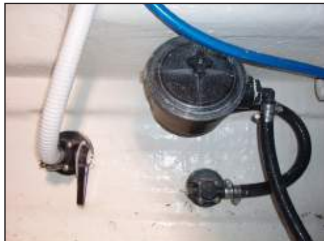
Holding Tank Overboard Discharge Thru-Hull Valve and Air Conditioner Sea Strainer
