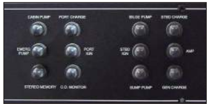
Battery Switch Breaker Panel
