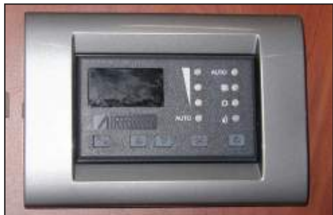
Air Conditioner Control Panel
