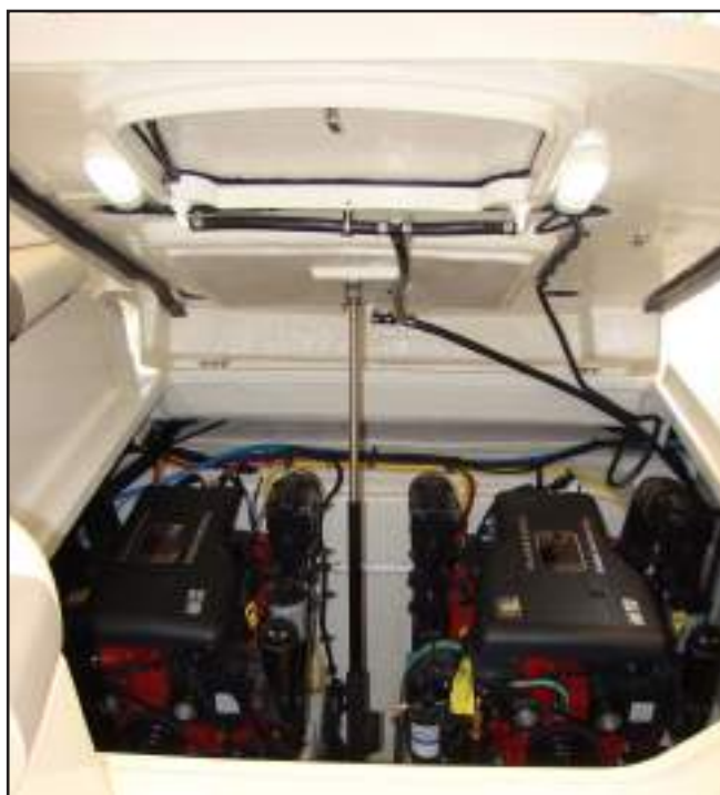
Engine Compartment Hatch, Day Hatch and Cockpit Drain System
