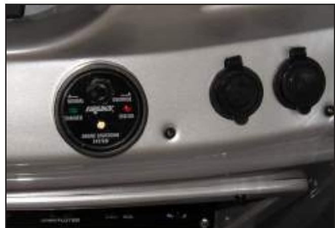
Override Switch and Fire Extinguisher Indicator Lights
