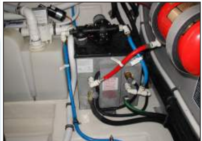
Fresh Water Pump, Water Heater and Waste System Vacuum Pump
