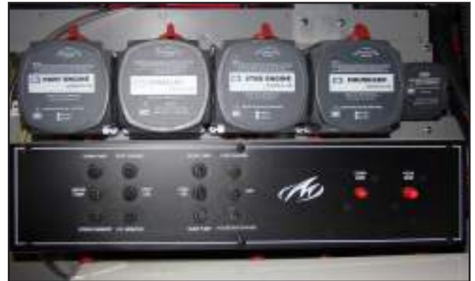
Battery Selector Switches, Circuit Breakers and Charging Relay
