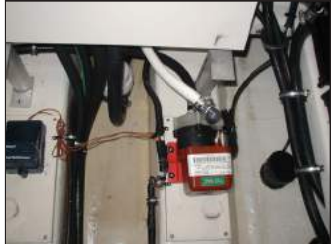
Air Conditioning Pump
