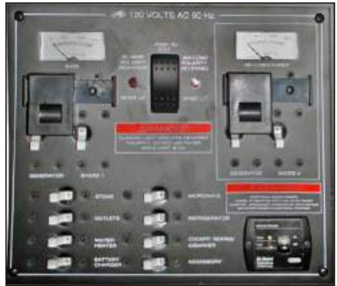
AC Accessory Breaker Panel
