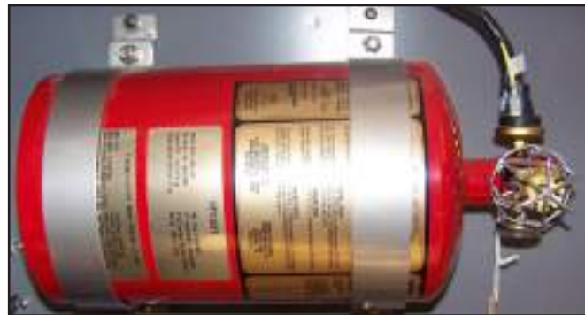
Automatic Fire Extinguishing System in the Engine Compartment
