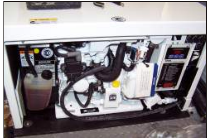
Typical Gasoline Generator
