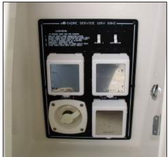
Shore Power Inlets, Breakers, TV/Phone and City Water Connection
