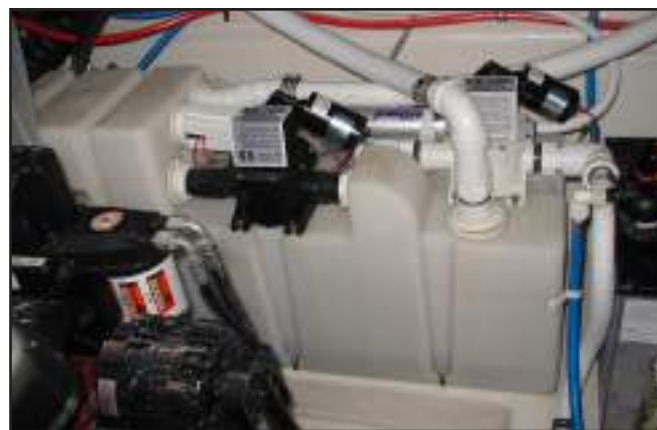
Holding Tank, Vacuum Pump and Overboard Macerator Pump
