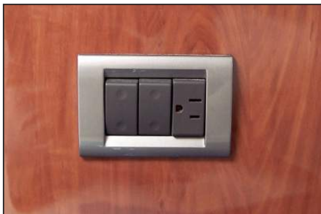
Typical Cabin Switch Panel and GFI Outlet
