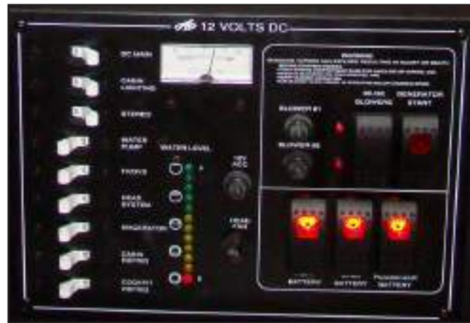
Cabin DC Breaker Panel
