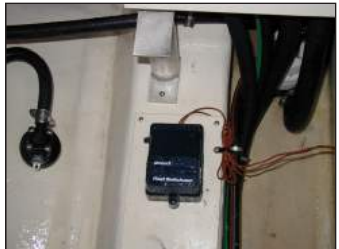
Automatic Float Switch for High Water Alarm and Emergency Bilge Pump Located Below the Engine Compartment Step.
