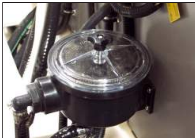
Generator Sea Strainer
