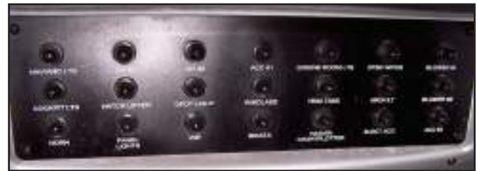
Helm Switch Breaker Panel
