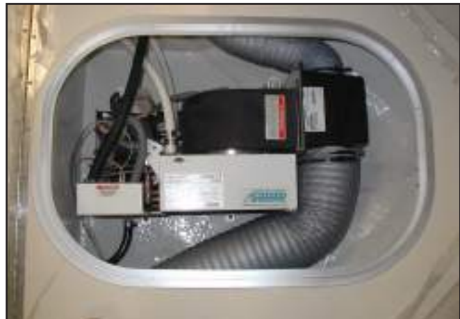
Air Conditioner Below V-Berth
