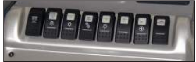
Helm Switch Panel - Port Side
