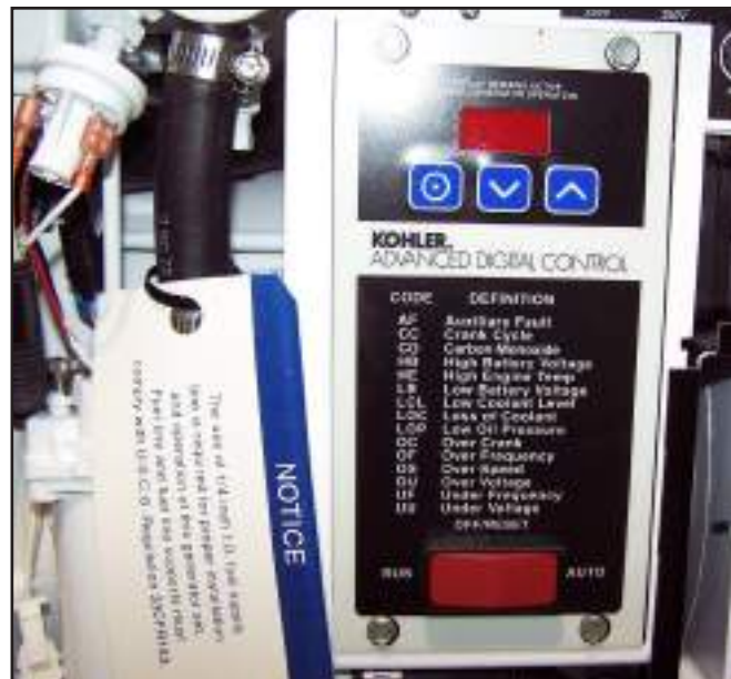
Generator Control Panel, Blower Switch and Blower Circuit Breakers
