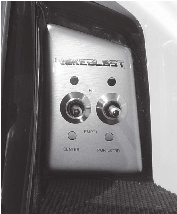
Figure B60: Ballast System Switch Panel
