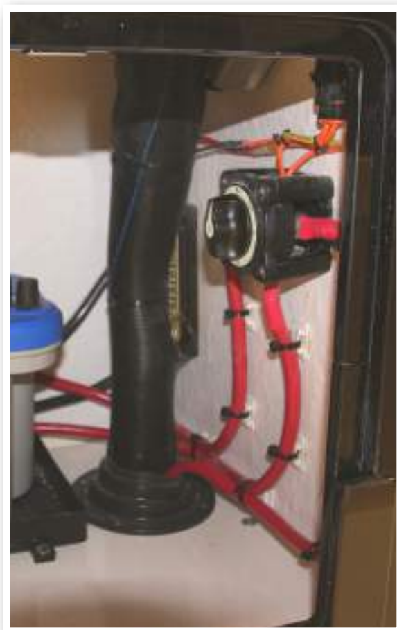
Battery Switch, Shown in the "Off" Position
