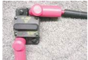
Figure 4-12. Main Circuit Breaker
