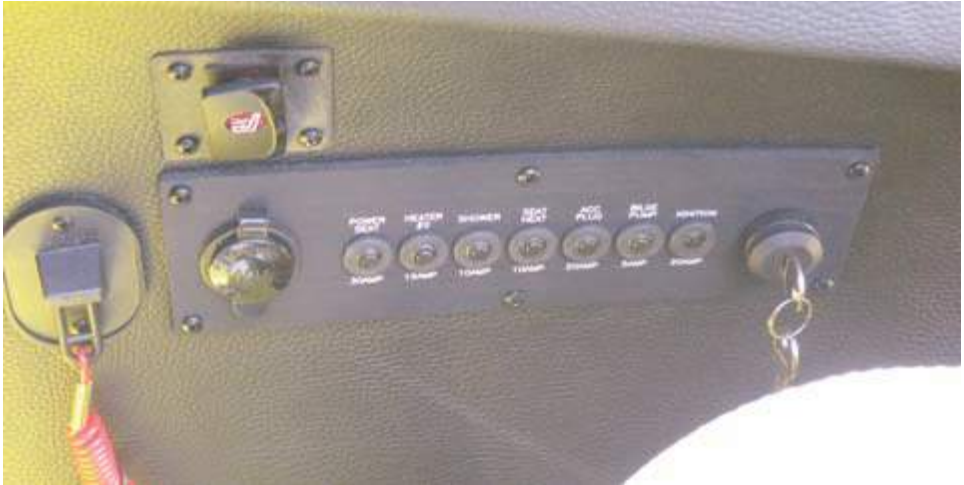
Figure 2-13. Circuit Breaker Panels
