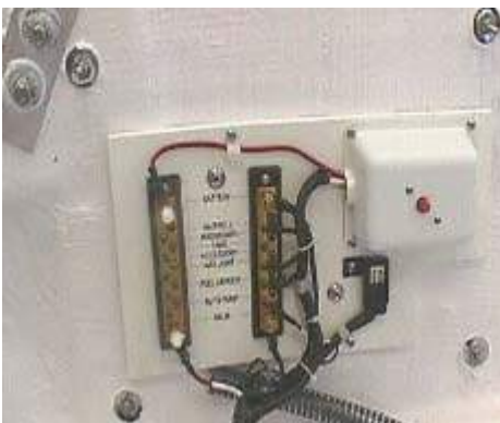
Positive terminal, Negative terminal, Main Breaker
