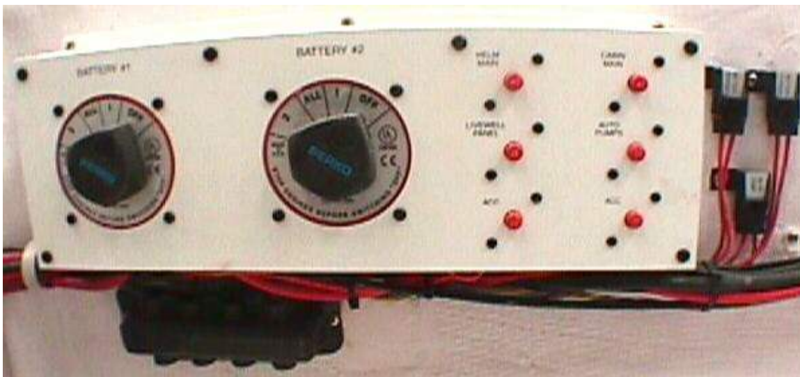
Bilge D/C Panel and Battery Selector Switches ^
