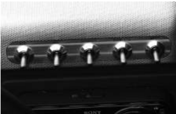
Figure H9: Helm Switch Panel - Starboard View
