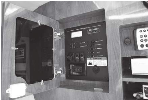
Figure H8: AC Power Panel
