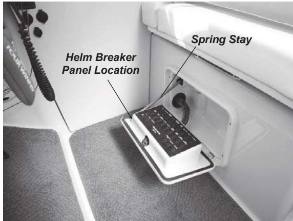
Figure H4: Helm Circuit Breaker Panel Location
