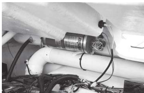
Figure L14: Optional Fire Extinguishing System
