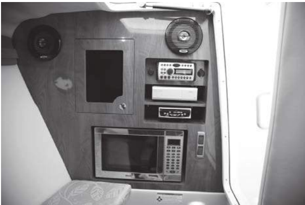
Figure Q1: Electrical Panel (Day Berth)
