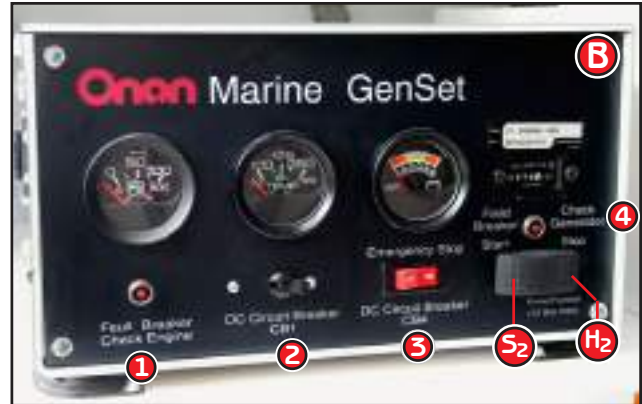
Onan GenSet panel
