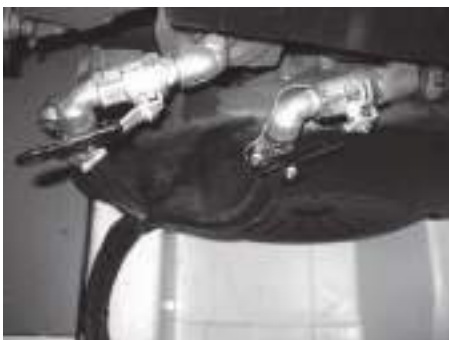
Supply valve port engine cooling system
