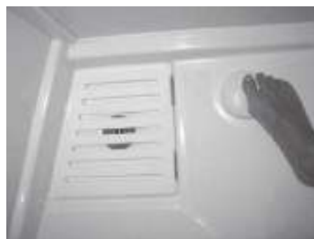
Control - Draining pump for shower
