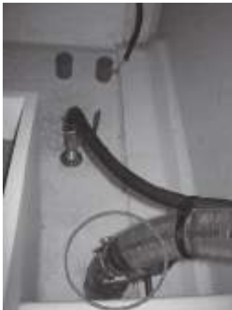
Sea water intake
