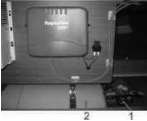
Water heater 220V- Access - Starboard aft cabin
