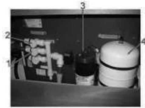
Plumbing board Saloon backrest
