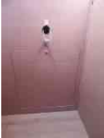
Location of the fire extinguisher port
