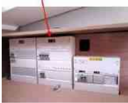
Ref 3: Differential switch (Operation)
