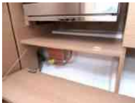
Gas supply valve
