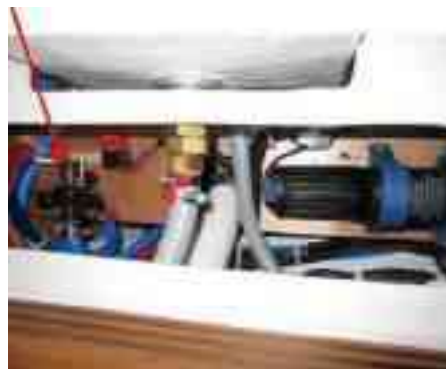
Electromagnetic valve Location: under the washbasin (Head)
