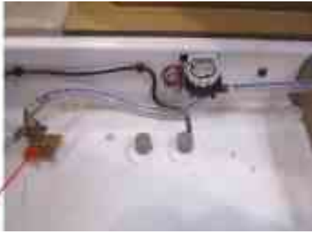
Sea water intake
