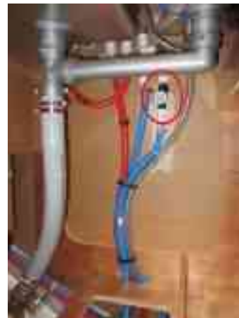
Fresh water socket Location: Under the sink
