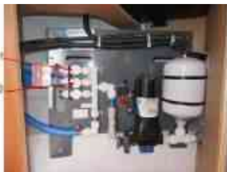
Water tank direction valves Location: Starboard saloon
