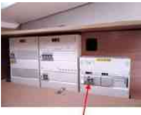
Converter circuit breaker Location: Port aft cabin
