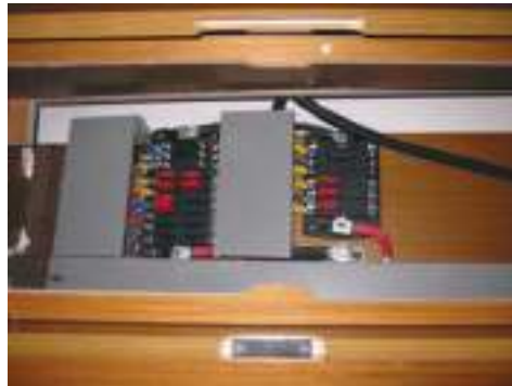
Fuse board - Back of electrical panel
