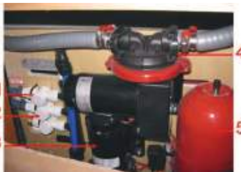
Plumbing board Saloon backrest Starboard
