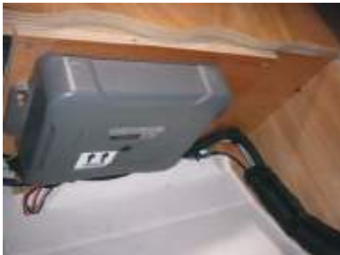
Vessel Management Unit - Bulkhead - Port aft cabin
