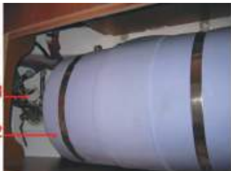
Water heater 220V- Saloon seating Starboard
