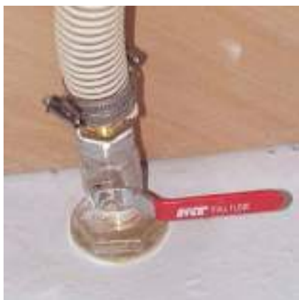
Thru-hull fitting closed
